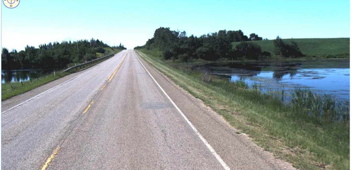
Sharp Edge and Steep Sideslope near Pond (Source: WebMap; km 13.921 looking South)
