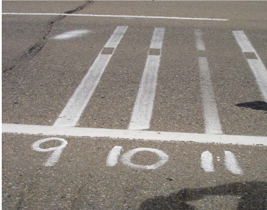
White paint, line #9 – 15mil, line #10 – 13mil and line #11 – 12mil The 12mil line (#11) is almost completely worn. The 13mil line (#10) is performing well.
