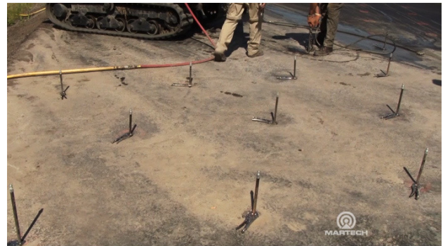
(a) Steel casing and probes were inserted into the ground in a 1.2 m triangular grid
