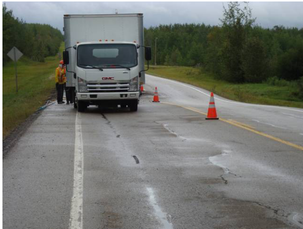
Figure 5. Settlement dip prior to foam column injection
