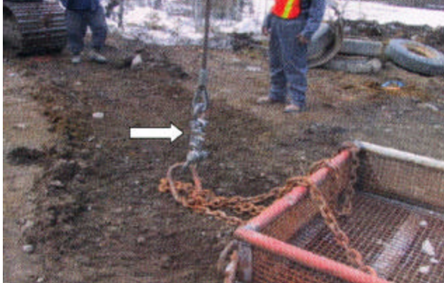
10-1 Load cell scale and hardware used to weigh heavy rock riprap at site
