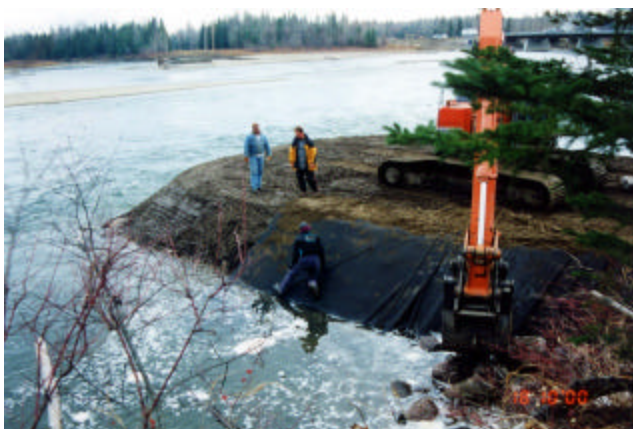
10-9 Placing filter fabric on well trimmed slope prior to placement of heavy rock riprap
