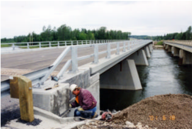
12-15 Bridgerail is the most prominent part of the bridge and its installation must result in alignment and elevation true to the required lines
