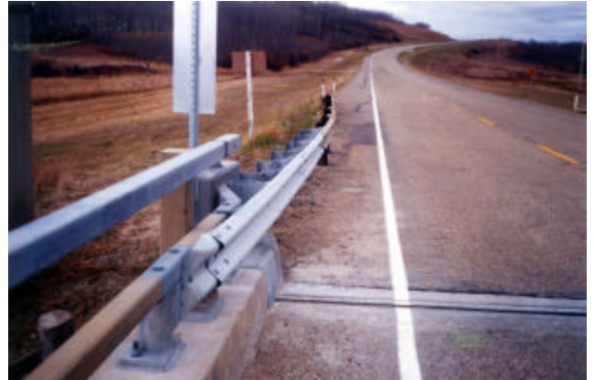
14-10 Realigning W-beam rail to shield the curb face at corner facing the direction of traffic
