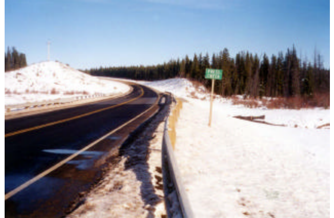
14-4 Looking northerly at SE corner approach guardrail has excessive curvature
