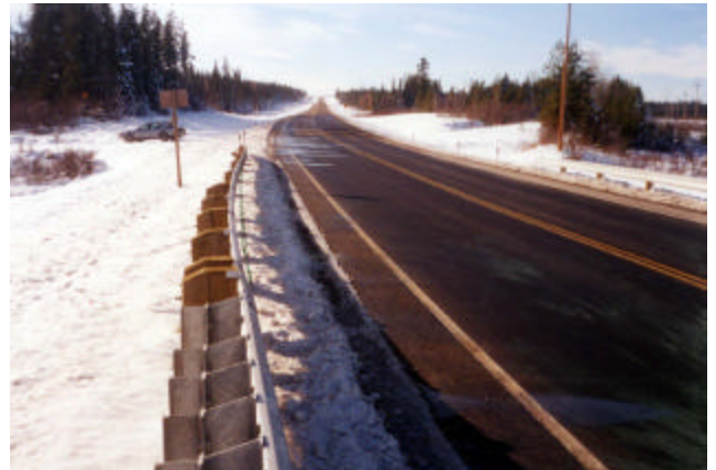
14-5 Looking southerly at SE corner approach guardrail has excessive curvature
