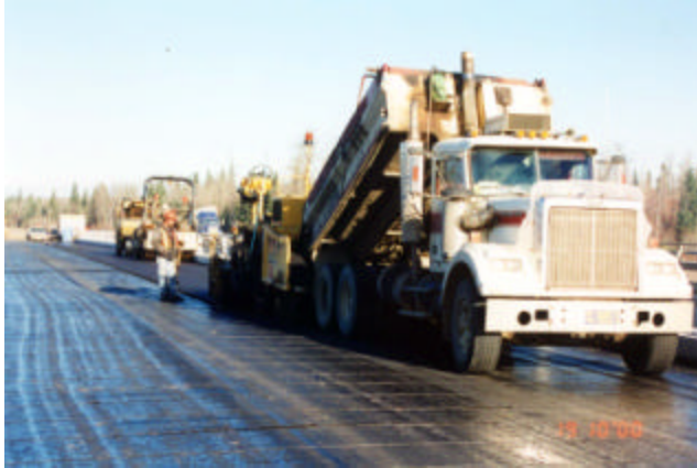
17-1 Placing the first lift of asphalt concrete pavement on waterproofing protection board
