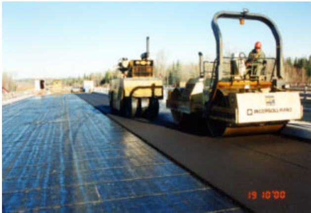
17-2 Compaction equipment: The first passes were made with a steel drum “knock down” roller, followed by a wobbly and finished using a steel finishing roller
