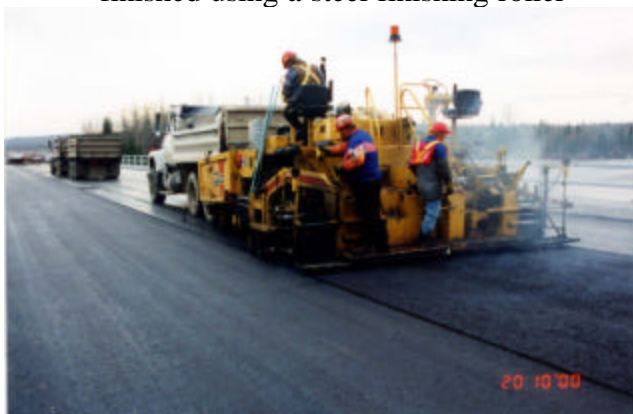
17-3 Placing centre mat on the final lift, the longitudinal paving joints were located outside the wheel path areas
