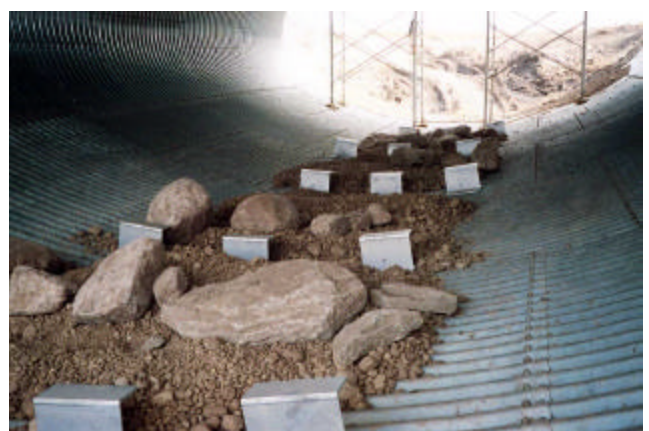
18-30 Randomly placed boulders on pitrun bedding. Fish baffles installed on culvert bottom
