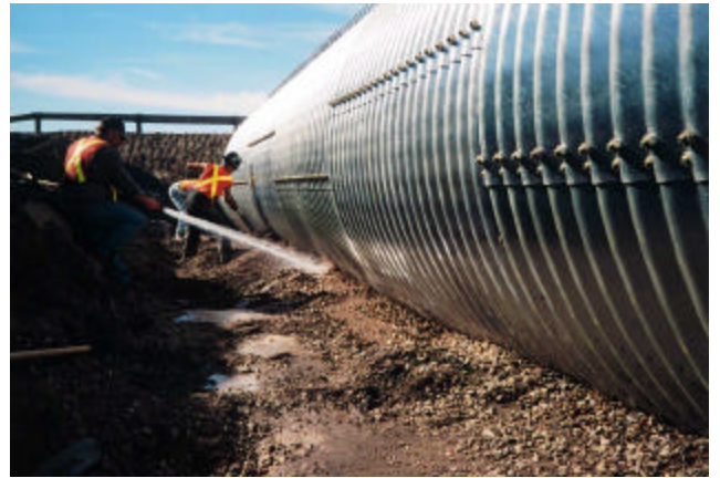
18-17 Improper way of water jetting material in haunches. Nozzle should be touching the haunch material
