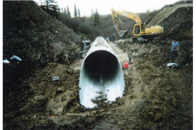
18-11 Bringing fill up on both side - Des. 2 Class 40 crushed gravel at barrel sections and clay seal on both ends of SPCSP
