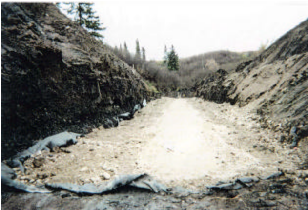
18-9 Bedding material – 150 mm lift of loose Des 2 Class 40 crushed gravel on 0.6 m of compacted Des.6 Class 80 pitrun on a layer of woven geotextile filter fabric
