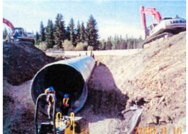
18-4 Bringing backfill up evenly at 150 mm lifts on both sides of the CSP
