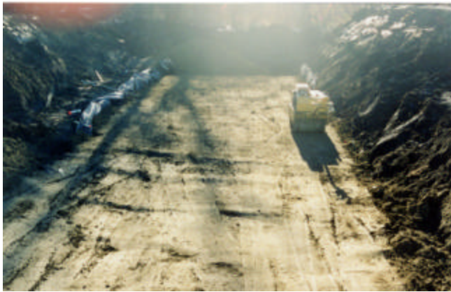
2-8 Backfill compact to 95% Standard Proctor Density at optimum moisture content with hand operated mechanical roller
