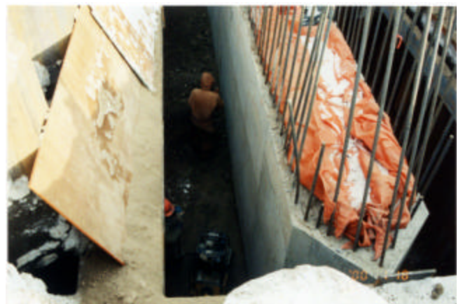
2-6 Backfill material placed in 150mm lifts and compact to 95% Standard Proctor Density at optimum moisture content with hand operated mechanical tamper
