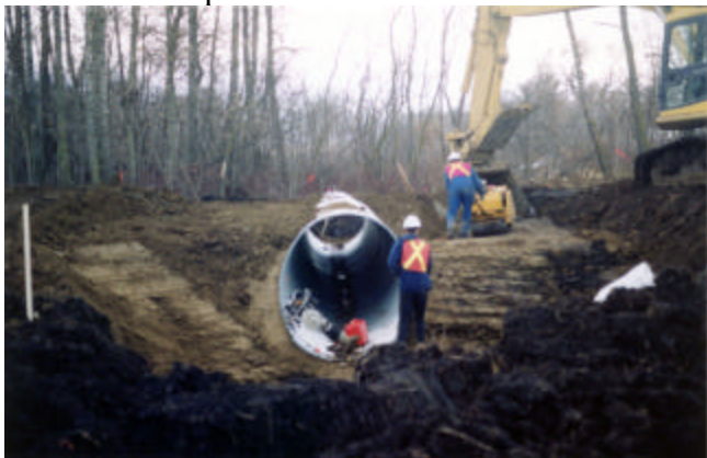
2-9 Bringing backfill up evenly on both sides of the culvert in 150mm lifts
