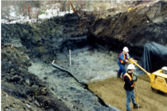
2-7 Backfill for culvert installation compact to 95% Standard Proctor Density at optimum moisture content with hand operated mechanical roller
