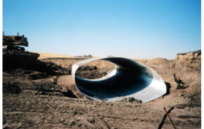
2-12 Bringing backfill up evenly on both sides of the culvert in 150mm lifts
