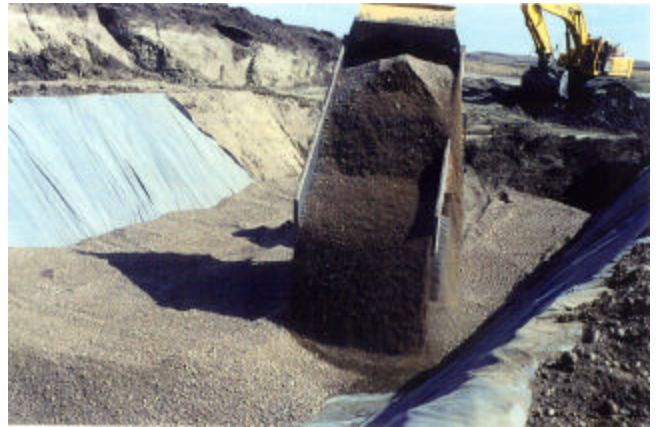
2-10 Culvert foundation (700 mm thick) Des. 6 Class 80 granular backfill compact to 95% Standard Proctor Density at optimum moisture content
