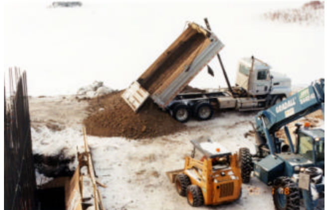
2-4 Granular backfill material delivered to site should contain no frozen lumps during winter months
