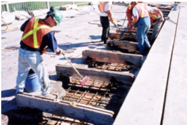
20-8 Preparation and forming of full depth repair prior to pouring of concrete.
