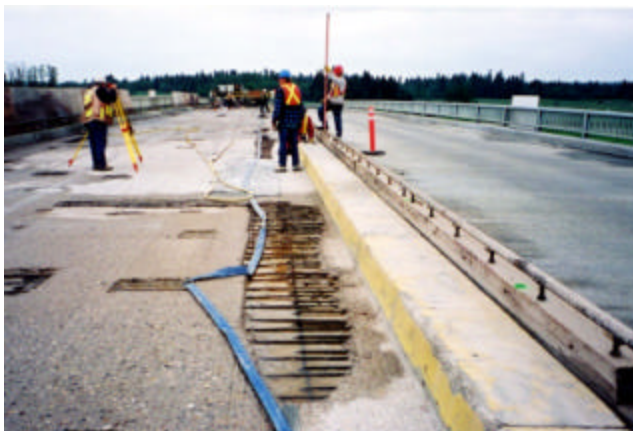
20-9 Full depth repair areas cast and cured prior to overlay concrete. Partial depth concrete placed monolithic with deck overlay concrete
