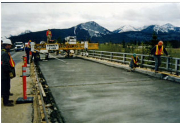
20-27 Fibre-reinforced concrete deck overlay is usually carried out on one half of the deck at a time, while traffic is maintained on the other half
