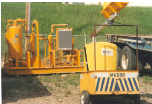
22-26 Air dryer and traffic control lights
