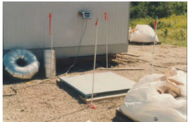
22-49 Pallet scale used to weigh sandblasting spoil contained in the bulk bags
