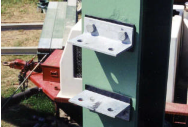
22-18 Galvanized bridgerail brackets are separated from painted steel by a neoprene gasket
