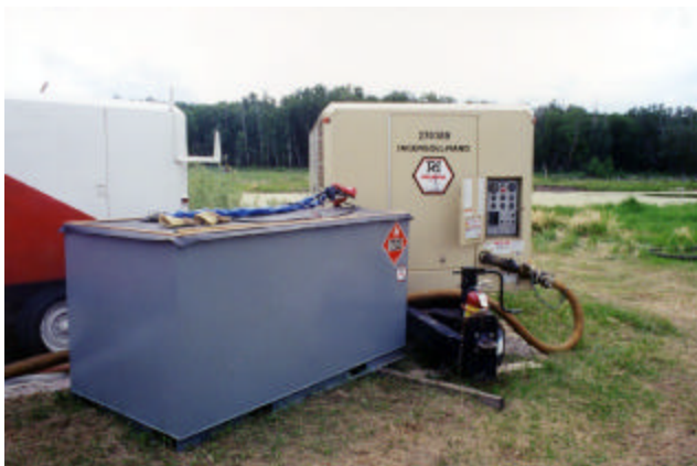
22-3 Air compressor and fuel tank
