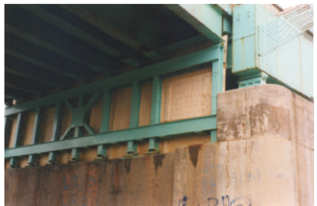
22-38 Plywood end panels containment structure are also used to protect steel surfaces not require painting
