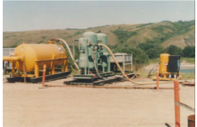
22-27 Air receiver and air dryer
