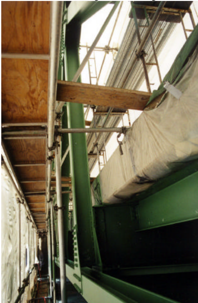
22-14 Non-paint area (curb concrete fascia) is protected against paint overspray with polyethylene sheet
