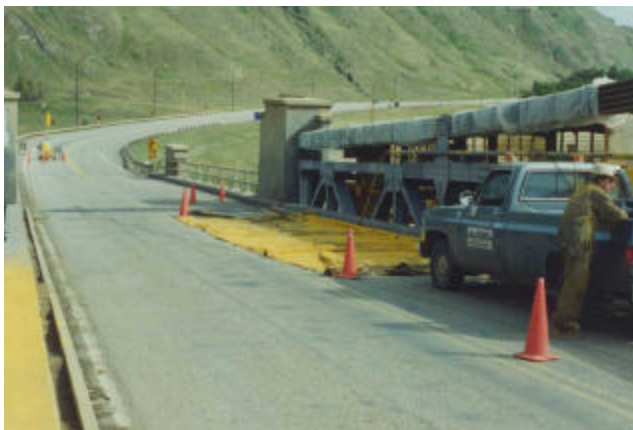
22-53 Protection of non-paint surfaces against paint overspray – clear polyethylene sheet wrap around main suspension cables and tarp lay on top roadway
