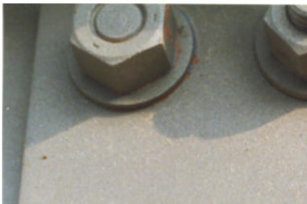
22-47 Bolt/nut areas are difficult to blast clean
