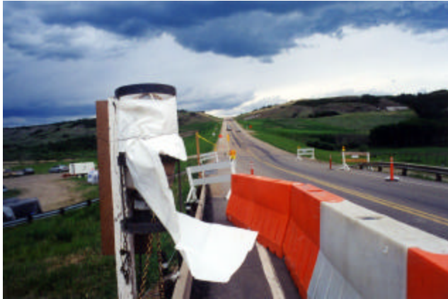
22-13 Polyethylene sheet wrapped around 1000w light to produce softer white light to avoid blinding the oncoming traffic
