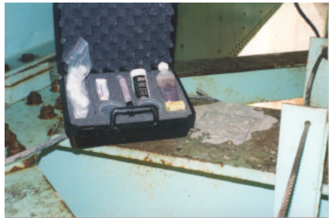
22-43 Scat kit used to check cleanliness after washing
