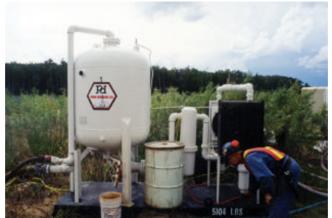
22-4 Moisture scrubber is used to remove moisture from air supplied by air compressor
