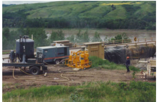
22-28 Sand pot, air compressor and air dryer
