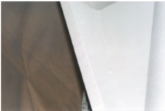
22-59 Blistering along edge of steel
