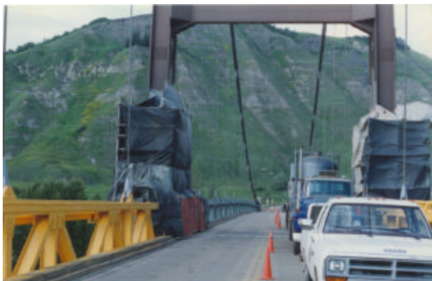
22-36 Tube and clamp scaffolding, reinforced tarp containment set up at lower portion of tower
