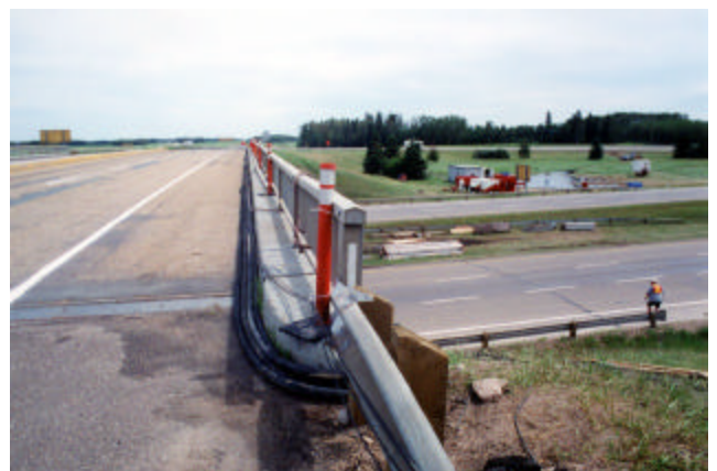
22-23 Multiple air hoses setup along curb for accessing various portions of the bridge
