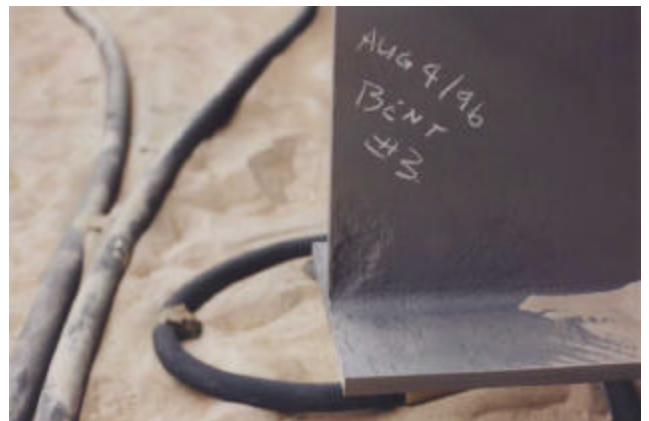
22-44 Beam blasted to SP6. Note sandblast spoil accumulated on platform floor
