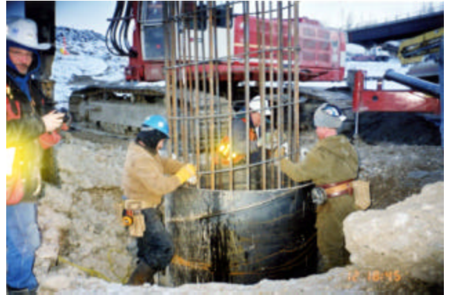
3-37 Placing reinforcing steel cage after hole has been satisfactory cleaned and inspected
