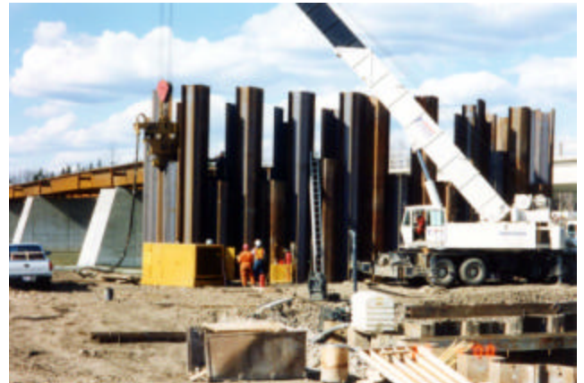
3-13 The first sheet pile for a cofferdam should be advanced one metre
