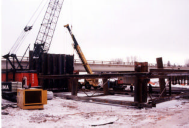
3-10 Two sheet pile driving frames were used to ensure sheet pile alignment
