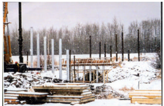
3-9 Diesel hammer driving pier pipe piles first and then driving abutment H-Piles
