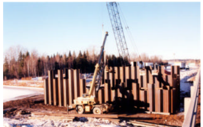
3-14 Subsequent piles advanced the same amount rotating equally from pile to pile
