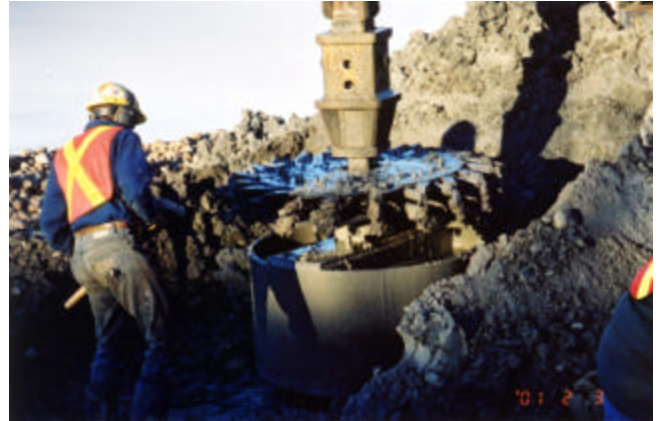
3-36 Cleaning sidewalls and bottom of drilled hole with wire brush/bucket drill rig attachment
