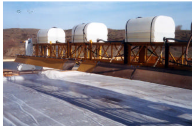
4-23 Fog misting setup - 3-100 gallon water tanks mounted to Truss Work Bridge
