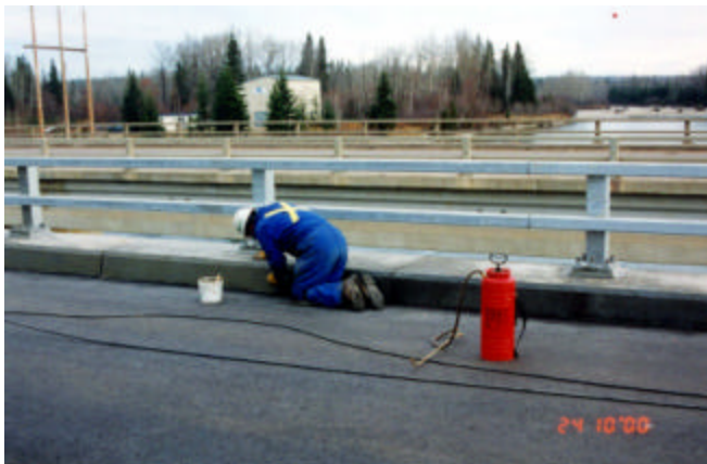
4-26 Curb face saturated with water for a period of not less than 30 minutes prior to rubbing with cement mortar
