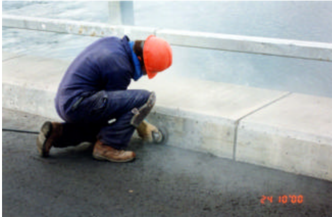
4-25 Grinding fins and irregular projections on curb face
