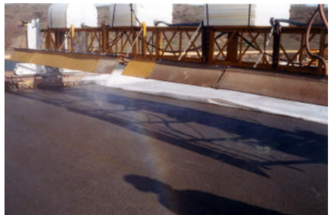
4-24 Fog misting being done over finished concrete prior to applying filter fabric curing material
