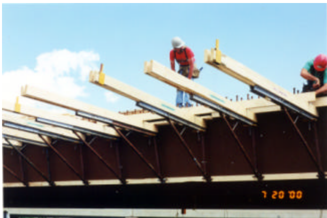
4-9 Deck form soffit knee braces c/w softeners at contact points between the knee brace and the steel girder
