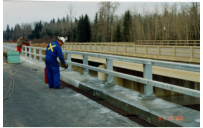
4-28 Applying sealer after curb concrete has been properly cured for at least 14 days
