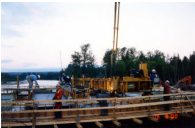
4-21 Work bridges immediately behind screed machine for bull floating and application of curing compound
