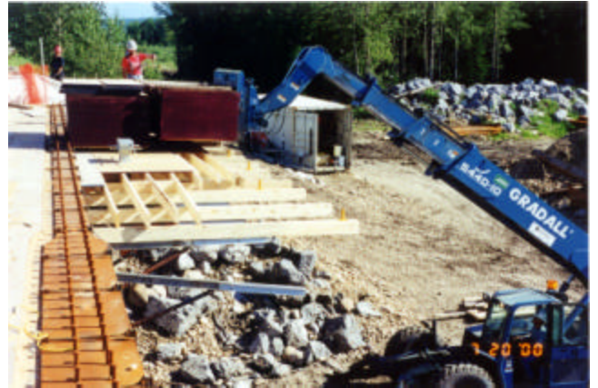
4-10 Load testing form taking into account the effect of form deflection under the actual construction loads
