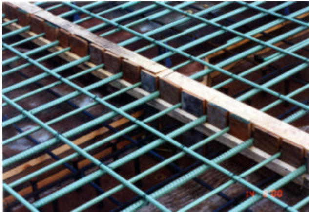
5-8 Bars tied at all intersections for spacing more than 250mm in each direction
