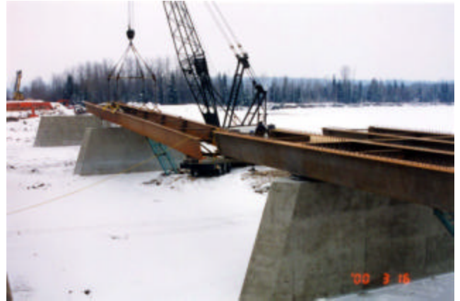
6-4 Winter frozen condition between piers permits one crane for erection of girder
