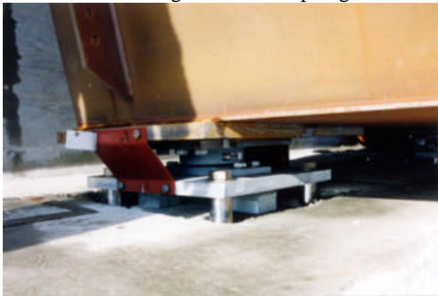
6-9 Bearing assembly supported on shim stacks
