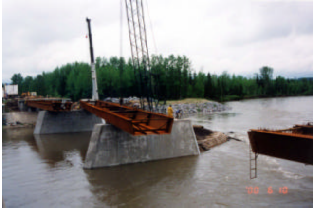
6-7 Summer open water condition requires two cranes and elaborate maneuverings to erect girders
