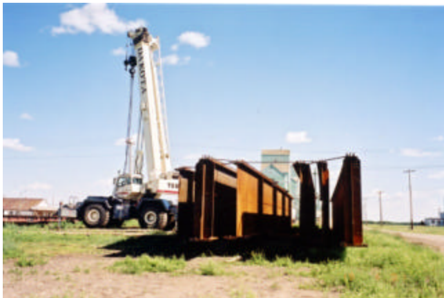
6-15 Steel plate girders off-loaded from railcar with braces installed to stabilize girders
