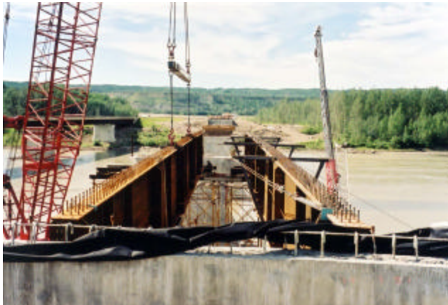
6-19 Steel plate girders are erected in pairs and are stabilized with steel diaphragms
