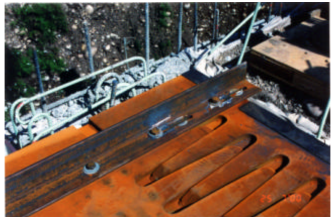
6-12 Deck joint gap set in accordance with the "Expansion Gap Setting Table"
