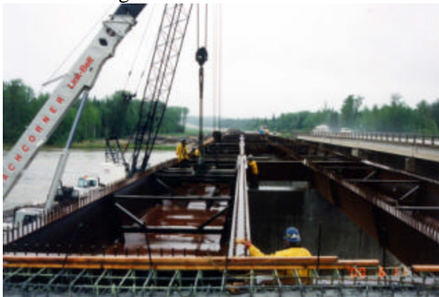
6-8 Summer open water condition requires two cranes and elaborate maneuverings to erect fill in girders and diaphragms
