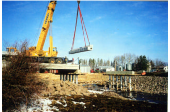
7-11 Erecting middle span girders on top of previously erected first span girders
