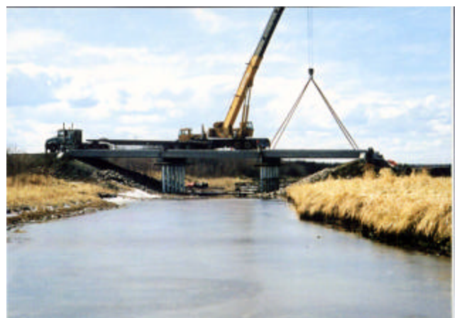
7-12 Erecting third span girders on top of previously erected middle span girders
