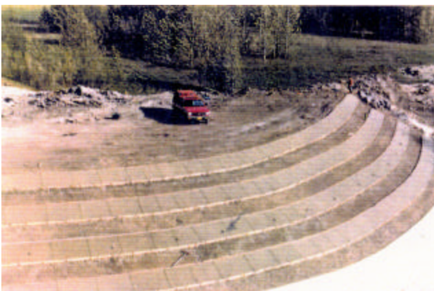
8-3 Pouring alternate strips to reduce shrinkage and control thermal cracking in addition to facilitating placing and finishing
