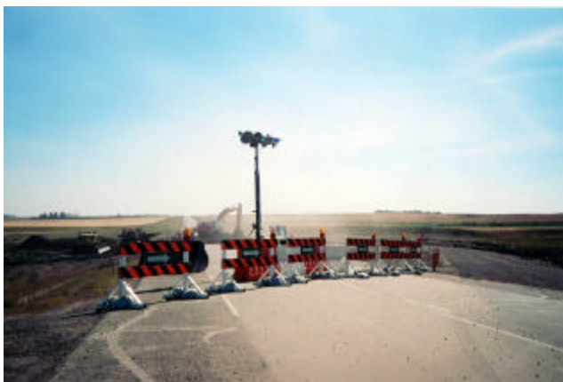
D-3 Site safety is enhanced with the placement of water-filled barriers and light towers
