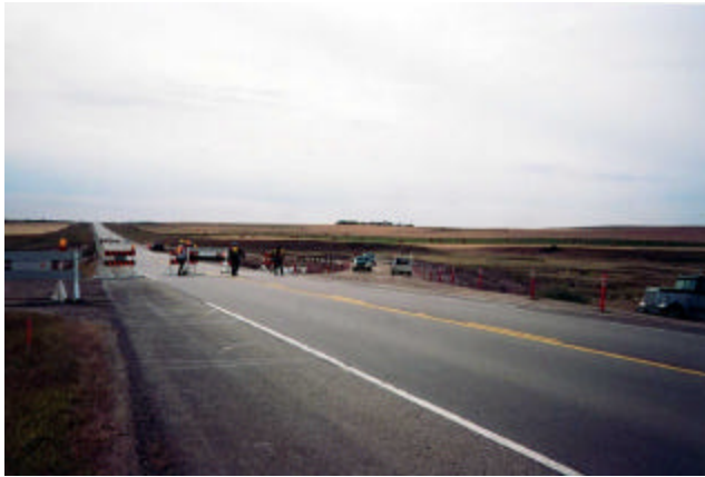
D-2 Blocking off highway with barricades, 2-way traffic are switched onto detour
