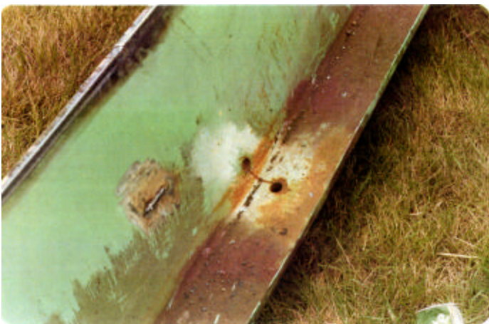
Drilling crack arrest holes in the flange and web can be effective in stopping the propagation of cracks – the far side of the flange is cracked across in the above photo.
