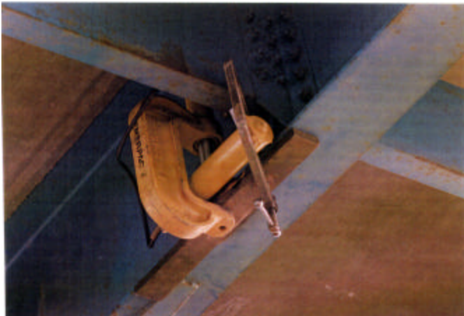
A hydraulic c-clamp used with heat straightening can be efficient in correcting localized flange distortions.
