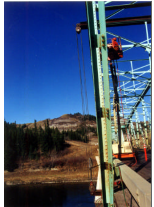
A truss tie may be required if repairs are needed for severely damaged tension members.
