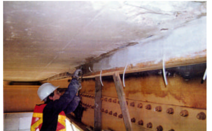
...loose concrete is removed, the haunch patched and the crack is epoxy resin injected. Installing injection ports.
