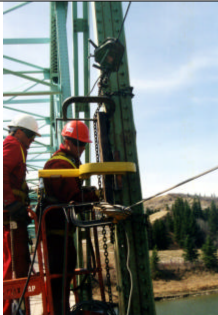
Effective heat straightening procedures may require several combinations of external force application with various heating patterns and techniques.
