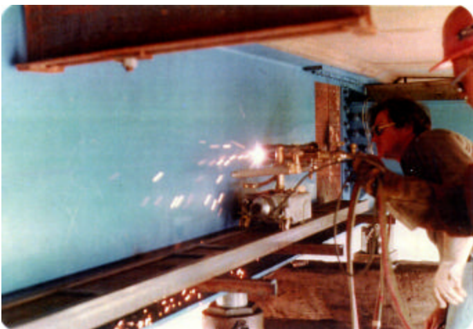
Severely damaged girder can be split and replaced with a tee girder section. A support track is installed, and a radiograph is used to make the section cut.
