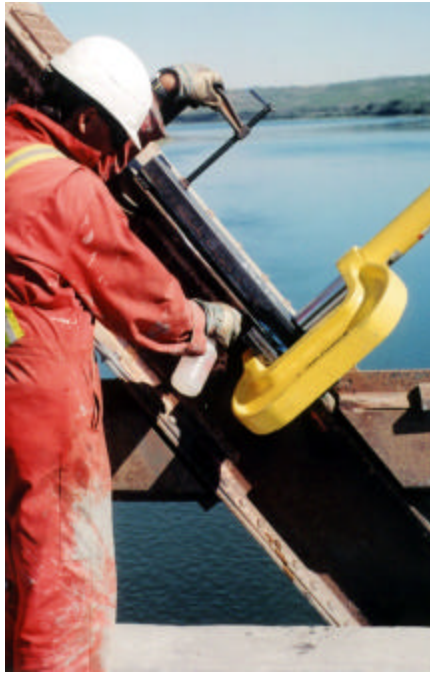
Applying water mist, after material has cooled below 315°C (600°F) allows more efficient time for heating cycles.
