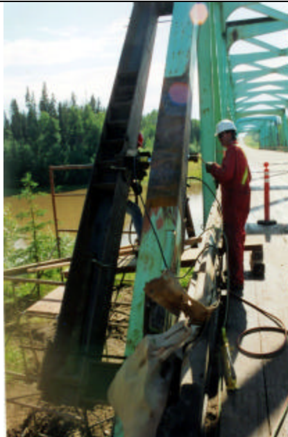
Jacking frames may be required to accomplish heat straightening effectively and efficiently in some circumstances.
