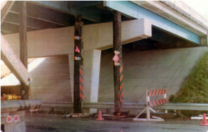
Intermediate temporary support blocking is required when the strongback deck support girders do not span pier substructure elements.
