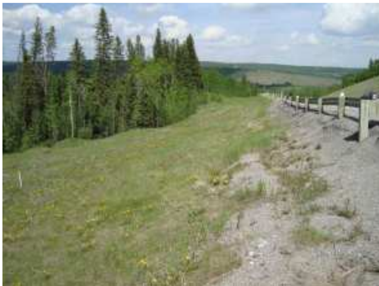
Photo S2-4 – Looking east at the slope below the highway in the landslide area. The slope appears to be in similar condition as was observed in 2009.
