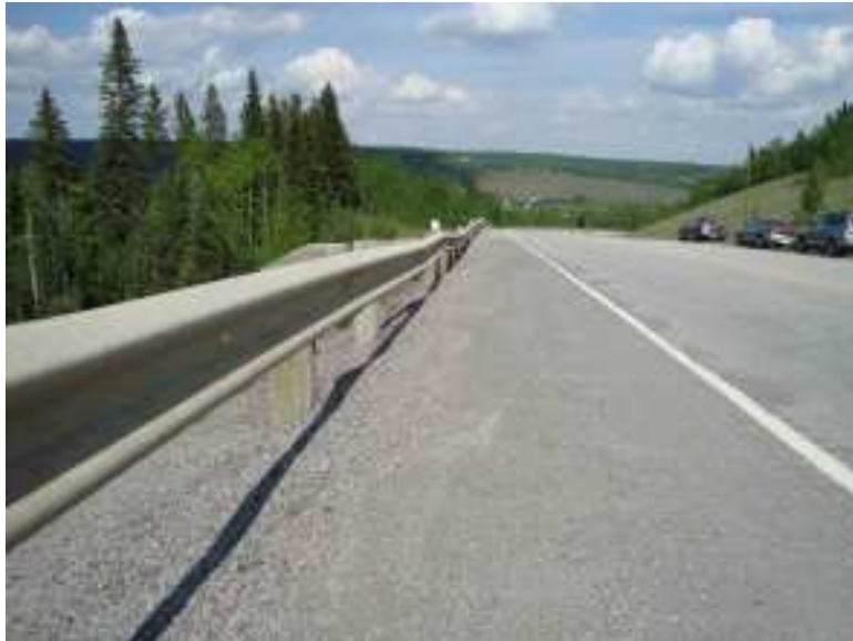
Photo S2-3 – Facing eastbound along the downslope shoulder of the highway from the west end of the landslide area. Settlement of the guardrail is visible in the area of the pile wall.
