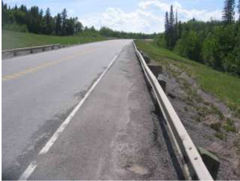
Photo S2-1 – Looking west along the downslope edge of the road along the pile wall area. Cracking in the road surface along the guardrail is present but covered with gravel and road debris. The road surface was in similar condition as was observed in 2009 and previous years with the cracking appearing to define the shape and extent of the existing pile wall.
