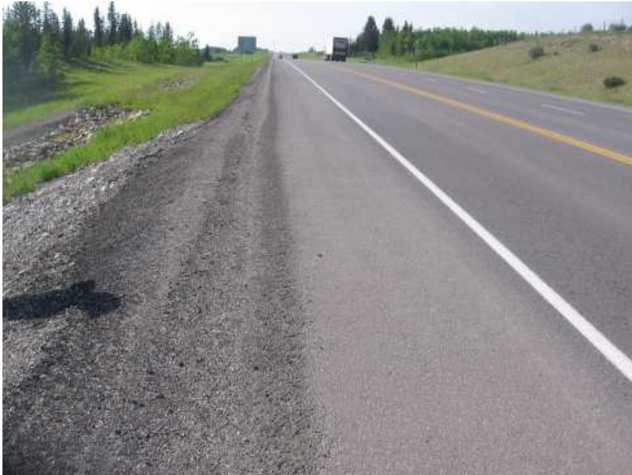
Photograph S3-1 – Facing southbound along the downslope shoulder of the highway, above the landslide area. An overlay was placed in this area in the summer of 2009 to repair past cracking and settlement of the road surface.
