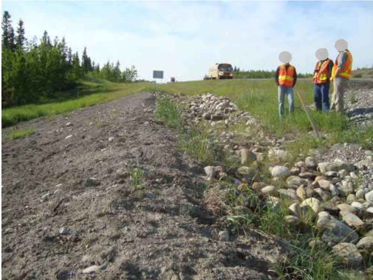
Photograph S3-2 - Looking southbound along the 2009 repairs to the ditch berm. Vegetation has not become established on the areas regraded in 2009.
