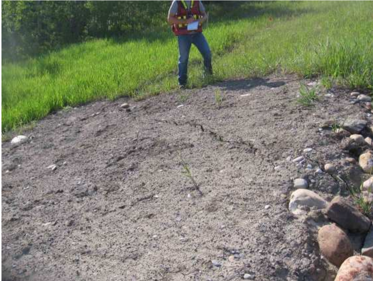
Photograph S3-3 - Crack formed at south end of the segment of the ditch berm that was regraded in 2009. The crack follows the same pattern as past damage, and likely indicates the south flank of the slide that remains active since the 2009 regrading.
