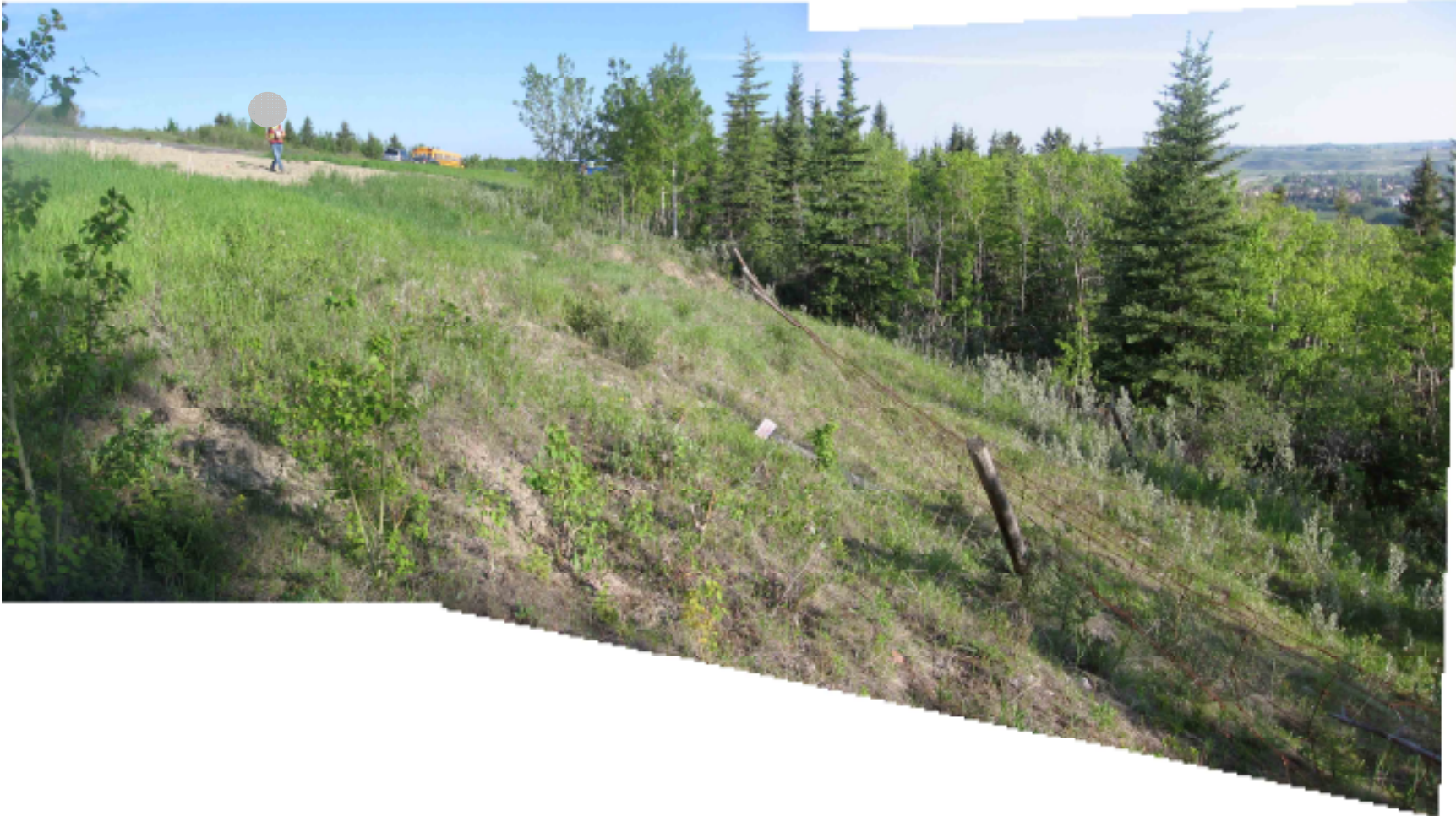
Photograph S3-4 – Looking northwest at the slope below the instrumented area. The condition of the tension cracks, slumps and fenceline damage have not changed significantly since the 2009 inspection.
