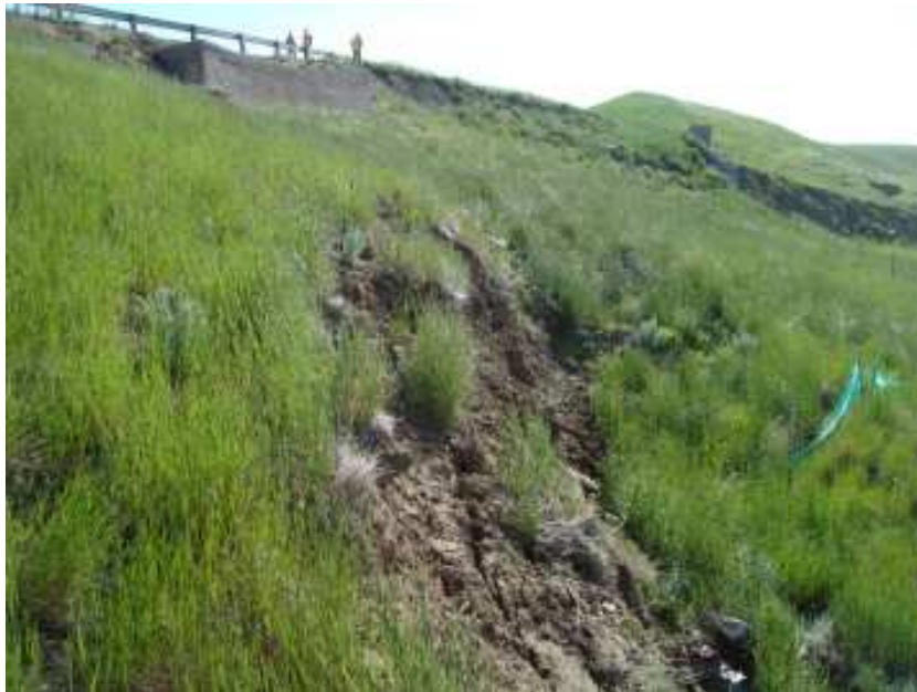
Photo S5-5 (top) Scarp recently formed on the colluvium slide mass below the retaining wall indicates continued movement of the slide mass.
