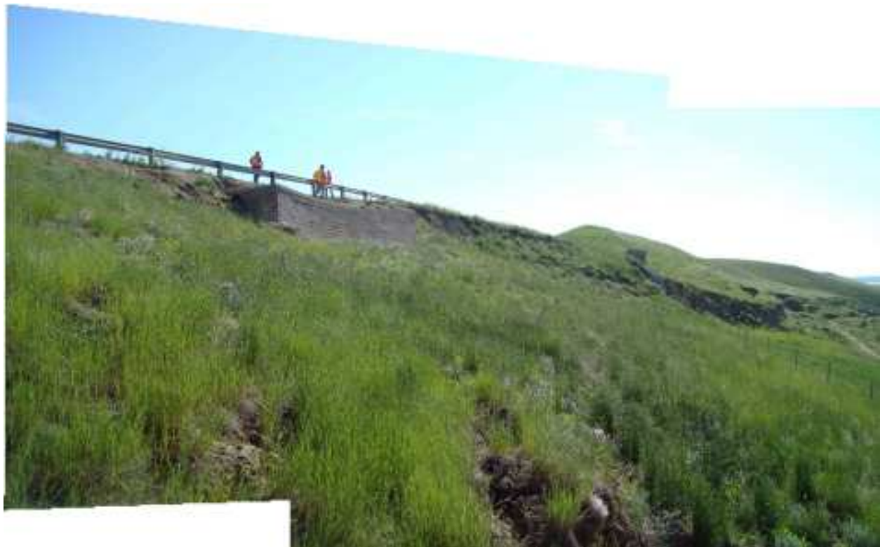
Photo S5-6 (bottom) General view of the site area from below the retaining wall.
