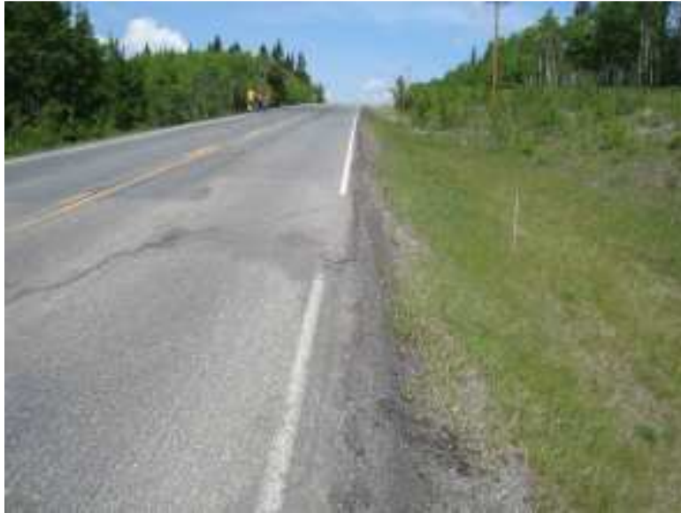
Photo S8-3 – Looking northbound along the east edge of the road near the centre of the site. No significant change to the road condition since the 2009 inspection. The road surface has been milled and this has revealed old cracks.
