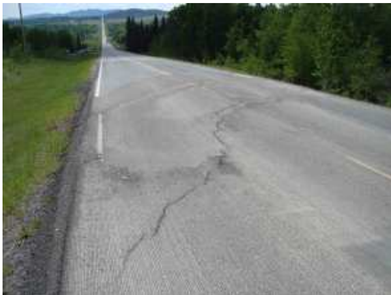
Photo S8-4 – Looking southbound along the east edge of the road at the south end of the site. No change to the condition of the road since the 2009 inspection. The road surface has been milled and this has revealed old cracks.
