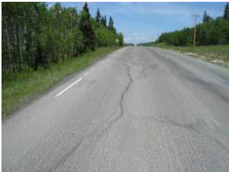
Photo S8-2 – Looking northbound along the west edge of the road surface at the north end of the site. The road surface has been milled and this has revealed old cracks.
