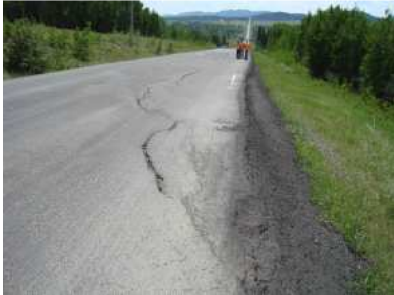
Photo S8-1 – Looking southbound along the west edge of the road at the north end of the site area. The cracking in this area follows the same pattern as has been observed in past inspections. The continued settlement and successive overlays has resulted in the asphalt becoming very thick, with a steep drop at the edge of the road. This area may require a guardrail. These cracks are likely old and have been uncovered by the recent milling, however some settlement has continued since the milling.
