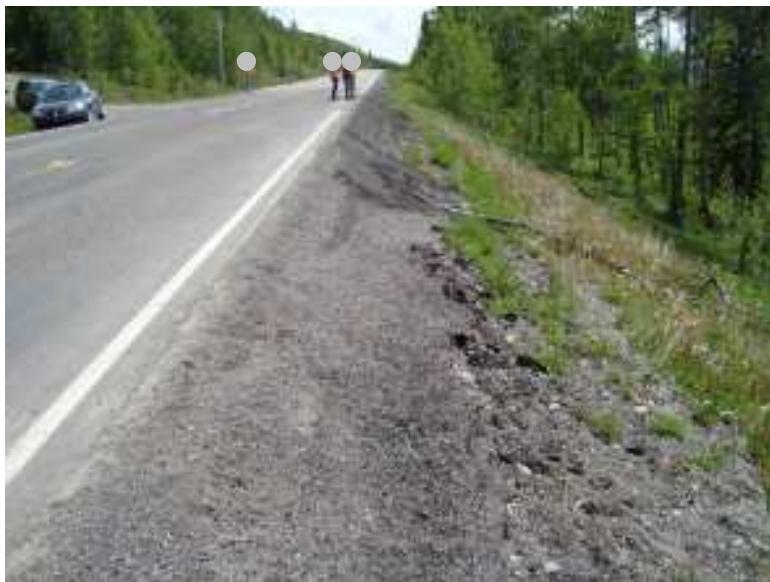
Photo S10A - 2 – Looking southbound from the north end of the site. Successive overlays have caused a steep drop to form at the edge of the road surface and have reduced the shoulder width. A guardrail may be required.
