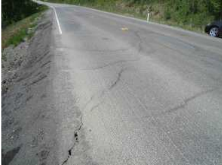
Photo S10A - 1 – Looking northbound from the south end of the site. The pattern and extent of the cracking in the road surface is similar to the conditions observed in 2009.
