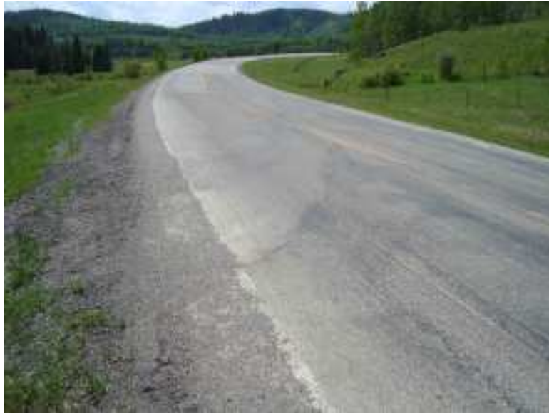
Photo S22-1 – Looking northbound from the east end of the site. The road surface has recently been milled which makes it difficult to compare the condition at the time of the inspection to past observations. The pattern and extent of the cracks in the road surface are similar to what was noted in 2009.
