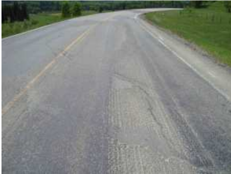
Photo S22-3 – Looking northbound from near the west end of the site. The cracking that has formed since the milling (or was exposed by the milling), follows the same pattern as past observation .s
