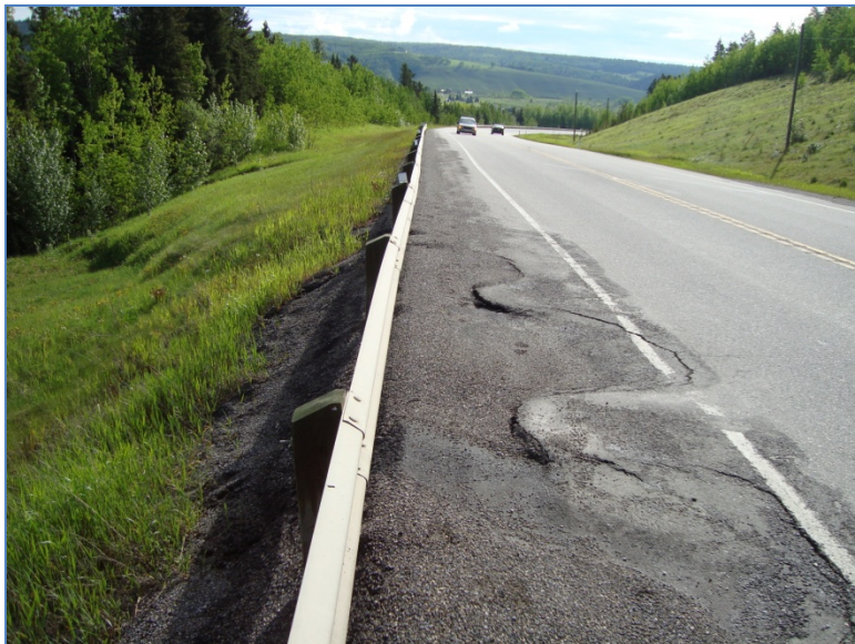
Photo S2-2 (June 2011) –Facing eastwards along the pile wall area. Cracking/settlement is visible up to the white line and the pattern of the cracking appears to delineate the existing pile wall.
