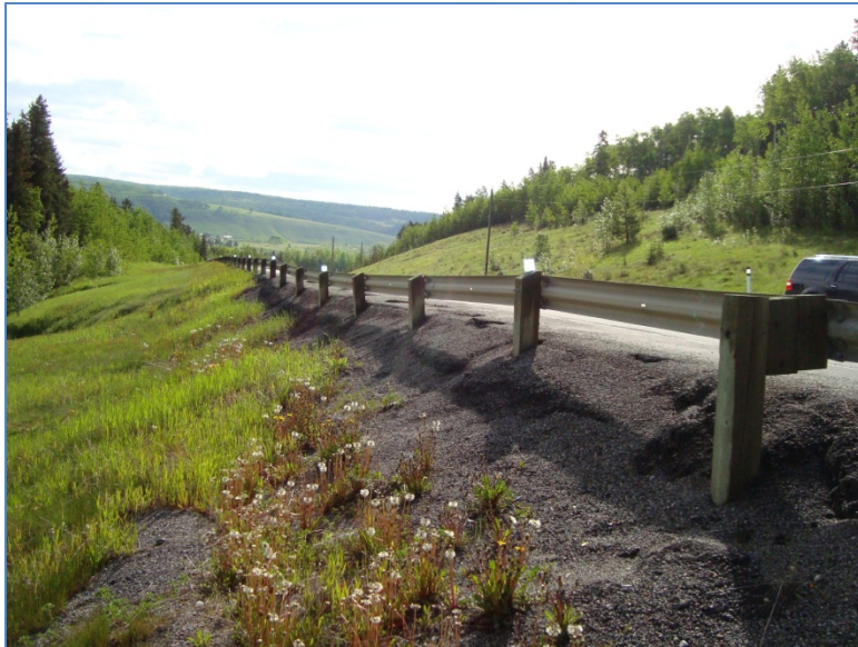
Photo S2-3 (June 2011) – Facing eastbound along the downslope shoulder of the highway from the west end of the landslide area. Settlement of the guardrail is visible in the area of the pile wall.
