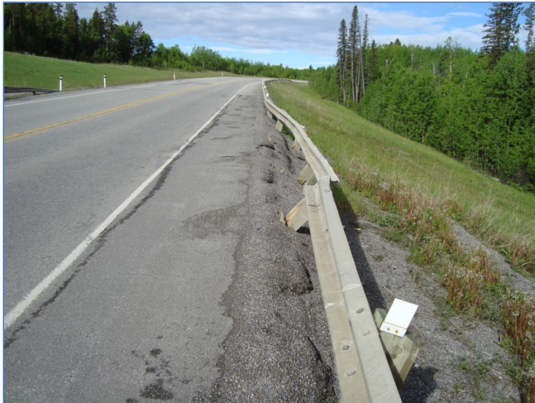
Photo S2-1 (June 2011) – Facing westwards along the downslope edge of the road along the pile wall area. Cracking in the road surface along the guardrail is present but covered with gravel and road debris. The road surface was in similar condition as was observed in 2010 and previous years. The guardrail was damaged due to a recent vehicle impact.
