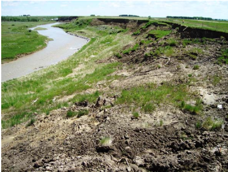
Photo S4-3 (June 2011) – Facing south at the slide area. Note the instability in the upper, steeper portions of the slope. Retrogression of the slide continues to occur with large blocks sliding down and adding to the slide mass.
