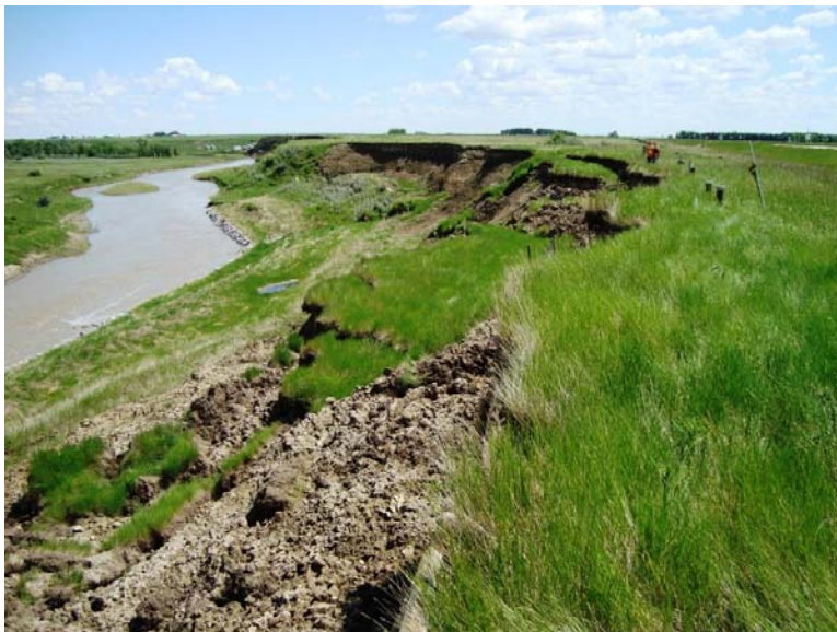
Photo S4-4 (June 2011) – Facing south at recent retrogressions of the slide scarp where large blocks have detached from scarp face. The blocks detached in late 2010 to early 2011.
