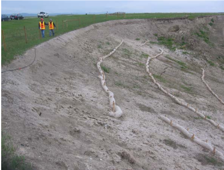
Photo S4-1 (June 2009) – Facing north across the soil nail repair area in 2009, for comparison with 2011 conditions (refer to Photo S4- 2).
