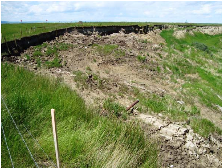
Photo S4-2 (June 2011) – Taken from the same location as Photo S4-1. Landslide movement has been ongoing, with continued retrogression at the slope crest and disturbance of the erosion control and bioremediation techniques by soil flows.
