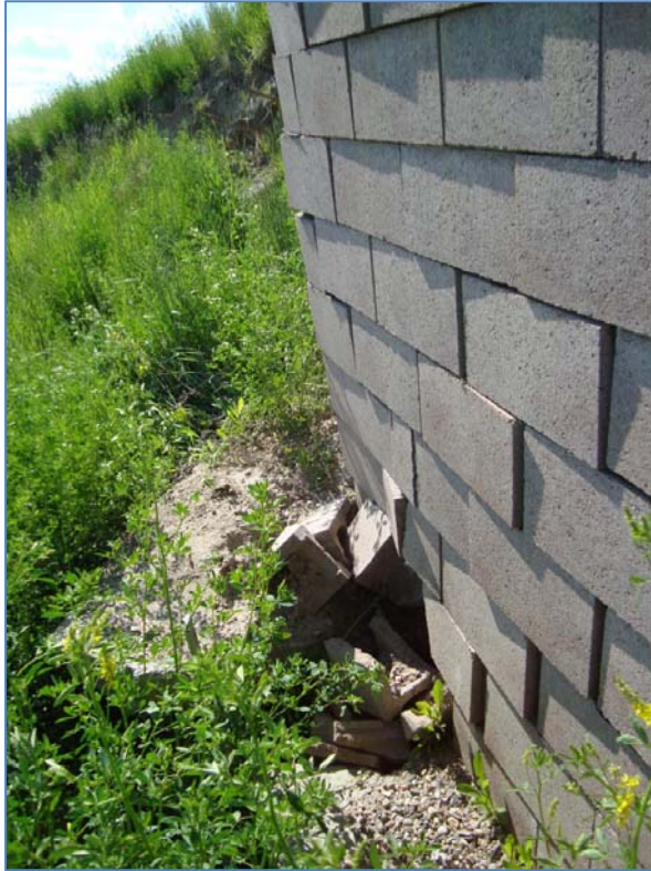
Photo S5-1 – top – (June 2011) The footing at the west end of the retaining wall has become undermined around the drainage pipe and cracking of the footing has occurred. The condition of the damage in this part of the wall has not changed significantly since the 2010 inspection.
