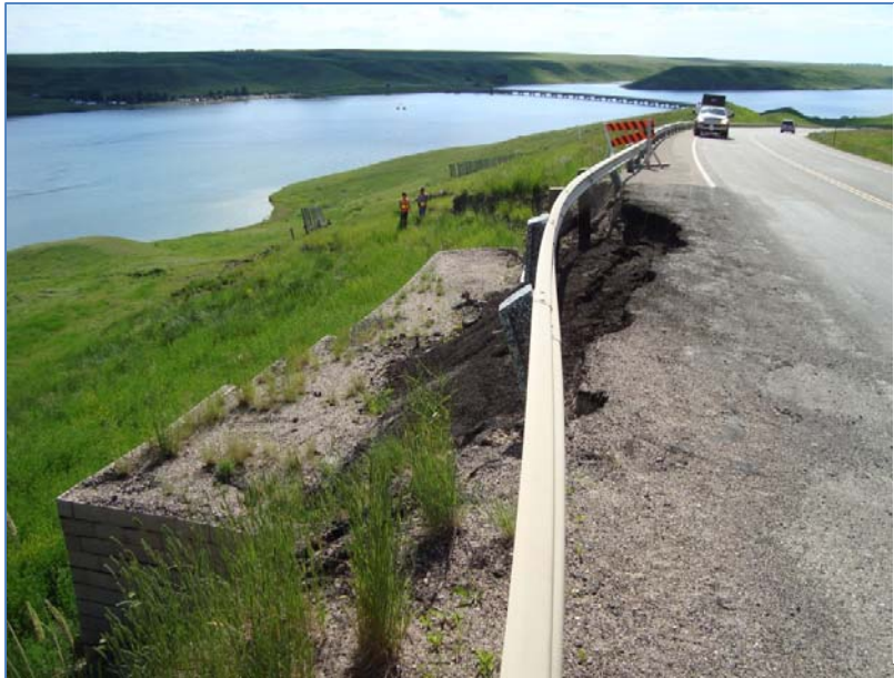
Photo S5-3 – top - (June 2011) Facing southwest at the retaining wall. The guardrail is visibly deflected, and the headscarp has retrogressed 1.3 m into the road surface.
