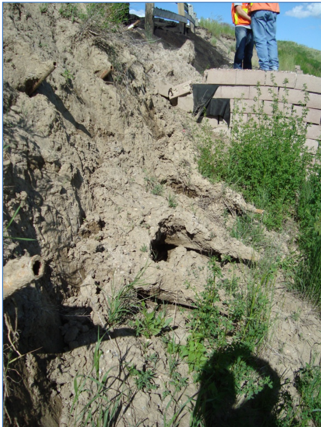
Photo S5-4 – bottom – (June 2011) Soil nails have become exposed at the headscarp.
