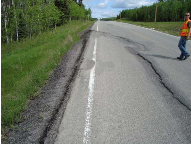
Photo S8-1 (June 2011) - Facing north along the west edge of the road surface at the north end of the site. This area had the most significant cracking at the site following a similar pattern as has been observed during previous inspections. The other areas of the site remained mostly unchanged since the previous inspection in June 2011.
