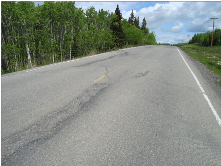
Photo S8-2 (June 2011) – Facing north from the middle of the site. The cracks in the road surface are relatively minor, and follow a similar pattern as has been observed during past inspections.
