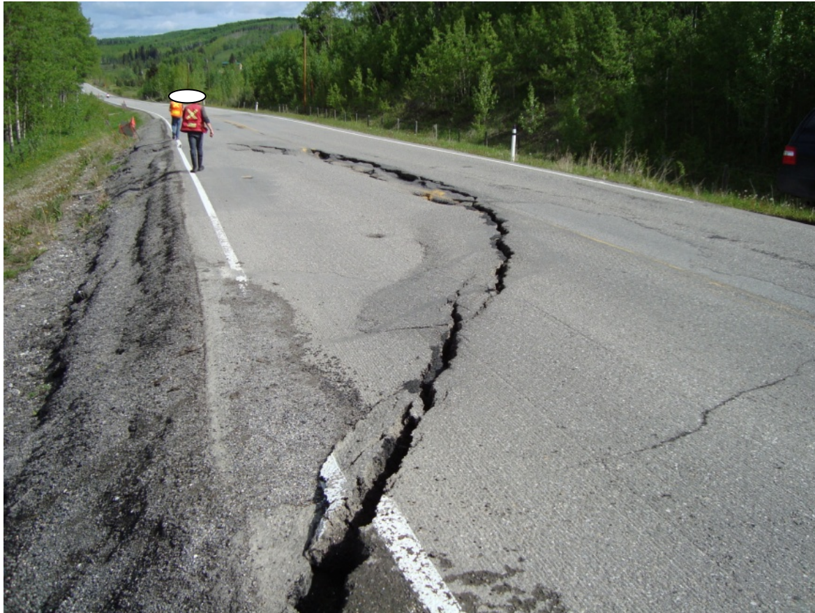
Photo S10A - 1 (June 2011) - Facing north from the south end of the site. The pattern of the cracking in the road surface is similar to the conditions observed in 2010; however, the magnitude of the vertical settlement and crack aperture has increased in comparison to the conditions during previous inspections.
