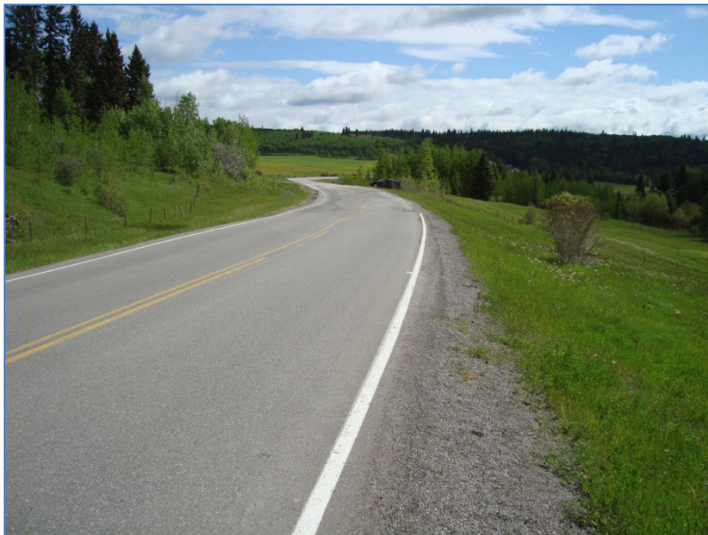
Photo S22-2 (June 2011) - Facing east (along the southbound lane) from the west edge of the site. The damage to the road surface is similar to that noted in past inspections.
