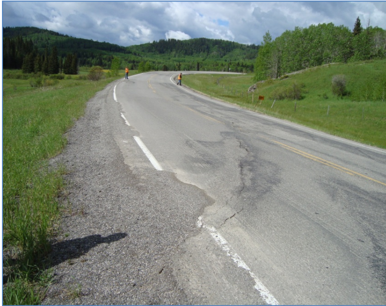
Photo S22-1 (June 2011) - Facing west (along the southbound lane) from the east end of the site. The pattern and extent of the cracks in the road surface are similar to what has been noted during past inspections.
