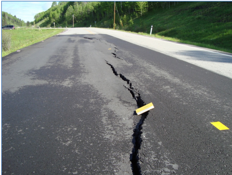
Photo S31-2 (June 2011) Close-up view of the cracking taken from the south facing north. The cracking has greater aperture and down-drop than the cracking measured during the previous inspections.
