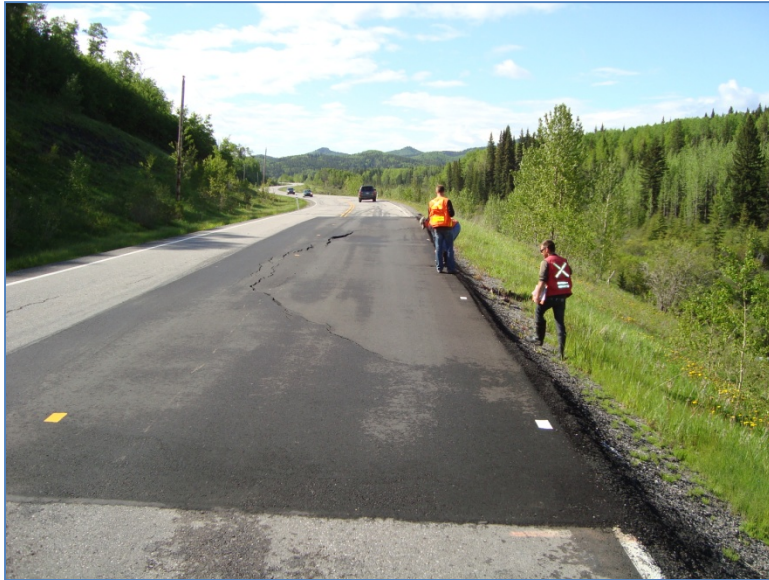
Photo S31-1 (June 2011) Facing south from the north end of the site. Cracking has developed through the recent overlay patch in a nearly continuous arc formed through the site area. This is the same pattern and extent of cracking noted during previous inspections.
