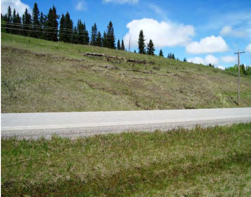
Photo 3 (May 2013) – Standing at the West Site looking towards the northeast at the backslope sliding.
