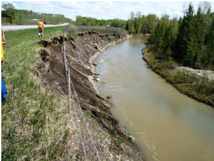
Photo 2 (May 2013) – Standing on the bank at the west end of the West Site, looking towards the east at the bank erosion.
