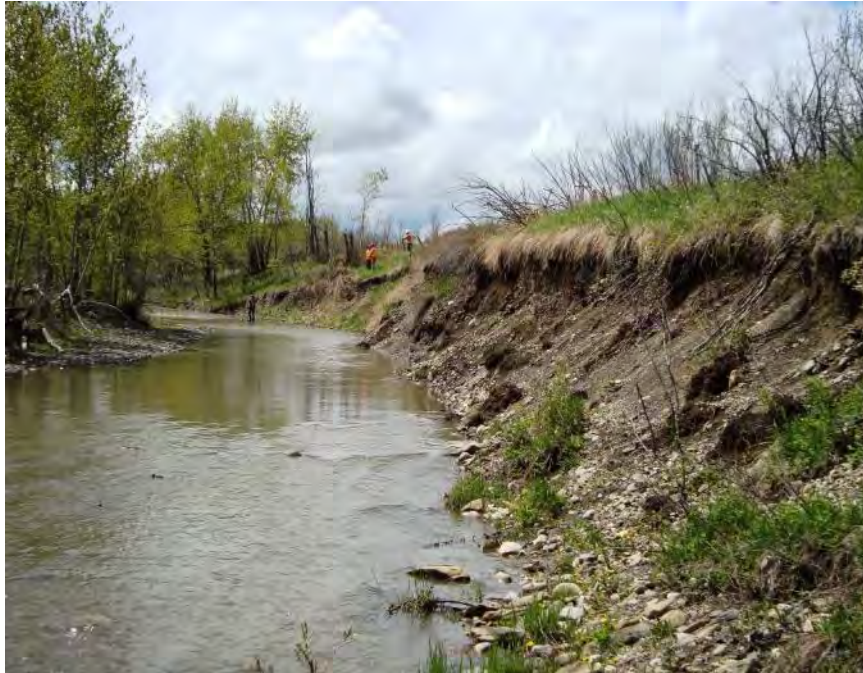
Photo 1 (May 2013) – Standing at the creek bank at the east end of the East Site, looking towards the southwest at the bank erosion.
