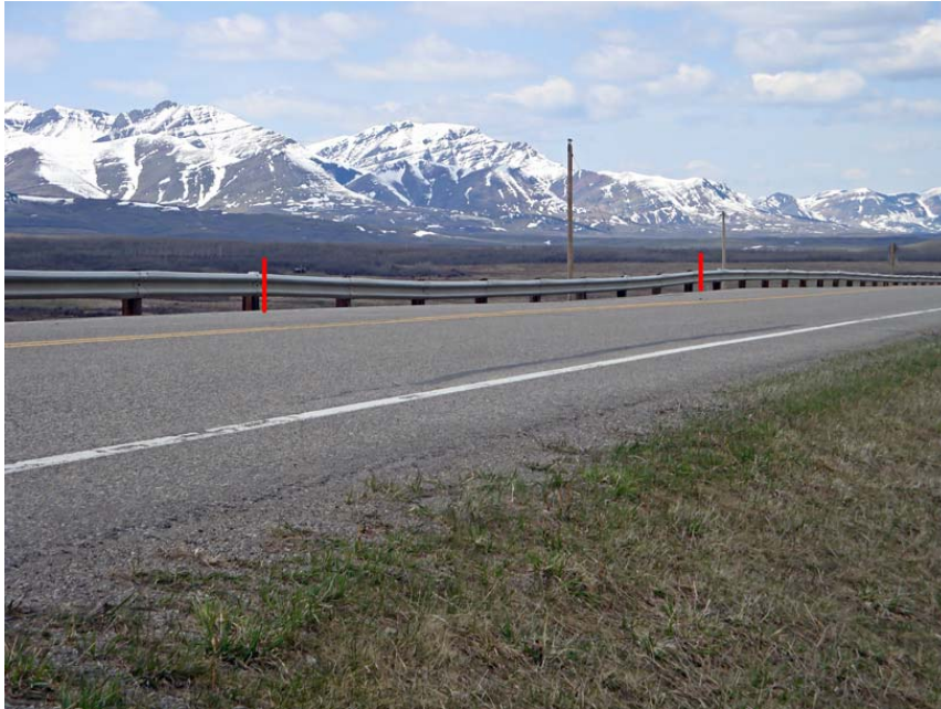
Photo S43-3 (May 2014) Standing in the upslope ditch looking towards the west at the slide area indicated between the two red lines. Note the settlement visible along the guardrail.
