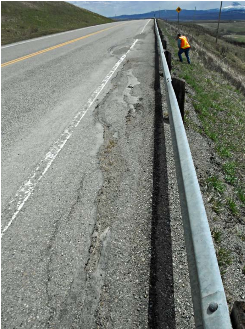
Photo S43-2 (May 2014) Standing in a similar location to Photo S43-1 and looking to the south at the cracking within the southwest road shoulder. The condition was similar to the 2013 inspection.
