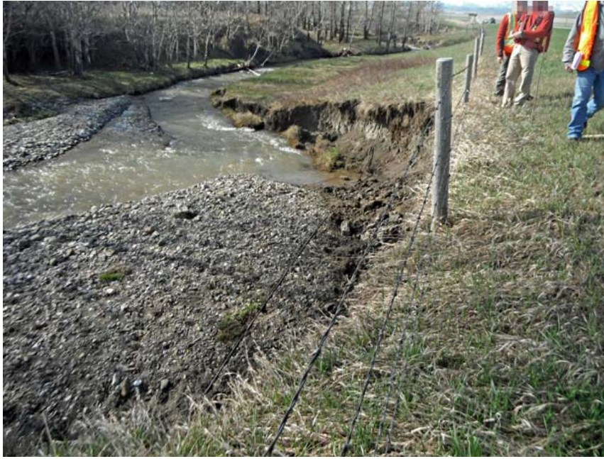
Photo S44-5 (May 2014) Photo of the same location as the previous photo (S44-4) during the 2014 annual tour. Increased erosion was observed but the minimum offset from the highway shoulder was unchanged. The creek flow had naturally channeled away from the bank in this area except at the south end, as seen here.
