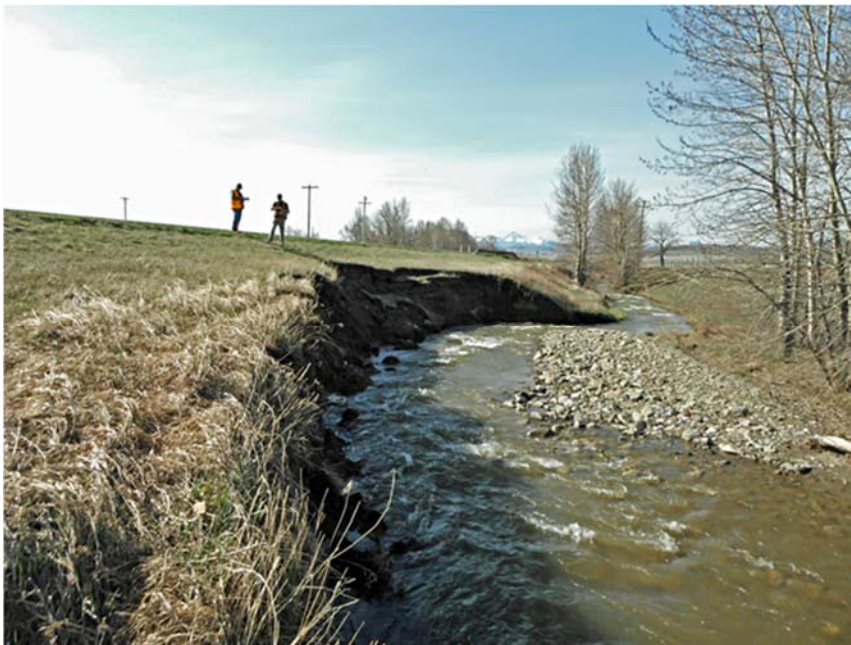
Photo S44-2 (May 2014) Standing at the same location as the previous photo looking south towards the encroachment area on the west embankment (Encroachment Area A1). There was increased retrogression and erosion visible against the bank relative to the 2013 conditions. The offset from the bank crest to the west road shoulder was approximately 3.8 m.
