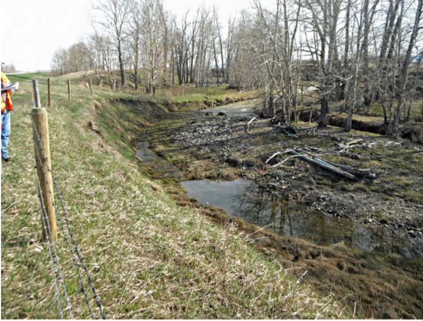
Photo S44-3 (May 2014) At Site B, standing on the east side of the highway embankment looking towards the northeast at Encroachment Area B1. Note the creek was not flowing in the old meander channel that had caused the original bank erosion.
