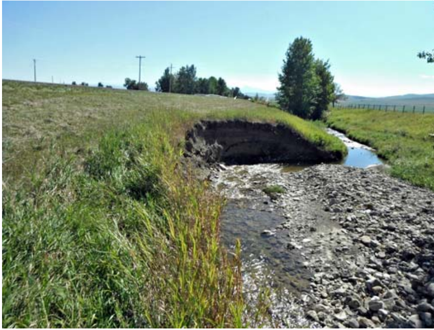
Photo S44-1 (September 2013) Standing at Site A on the highway's west embankment looking towards the south at the encroachment area. During the 2013 inspection the minimum offset from the bank edge to the road shoulder was approximately 6 to 7 m.
