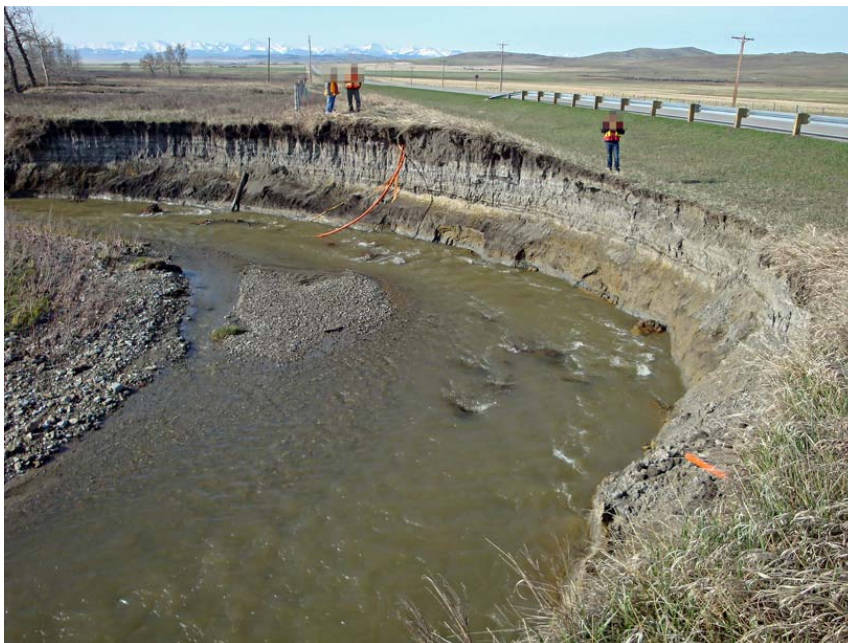
Photo S44-8 ( May 2014) Standing in a similar location as the previous photo looking towards the southernmost encroachment area as viewed during the Annual Inspection Tour in May 2014. Note the erosion of the previously fallen bank soils and new guardrail installment.
