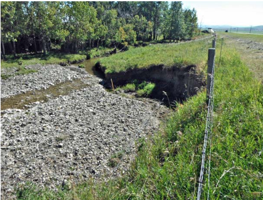
Photo S44-4 (September 2013) At Site B, standing on the east side of the highway embankment looking towards the south at Encroachment Area B2 in 2013. This area was previously referred to as the northernmost encroachment area at the South Site.
