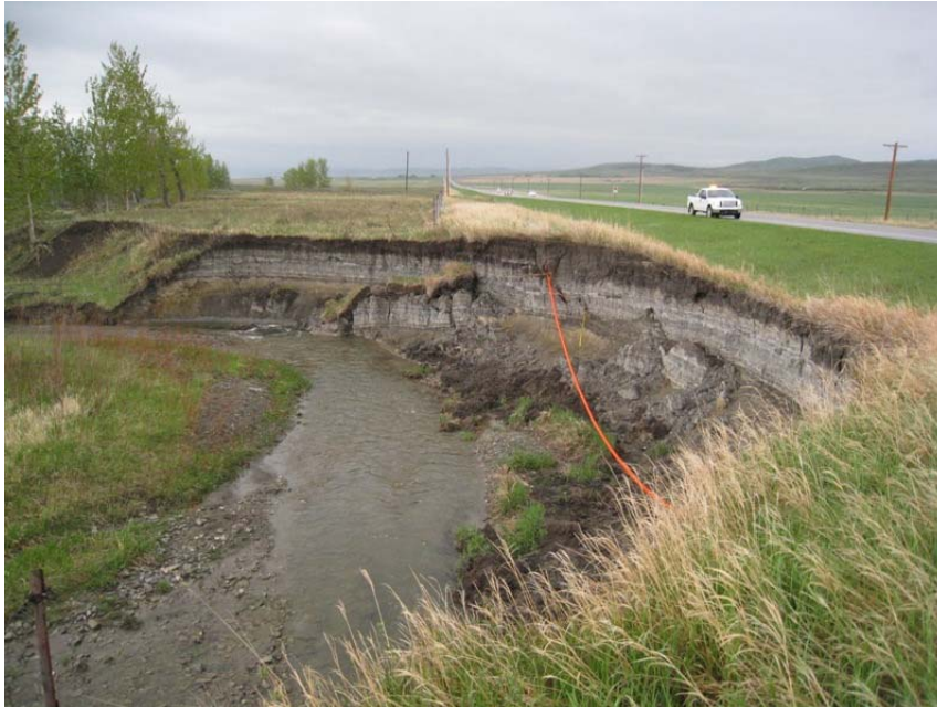
Photo S44-7 ( May 2013) Standing at the South Site on the highway's east embankment looking towards the south at the southernmost encroachment area. The site conditions as observed during the Annual Inspection Tour in May 2013.
