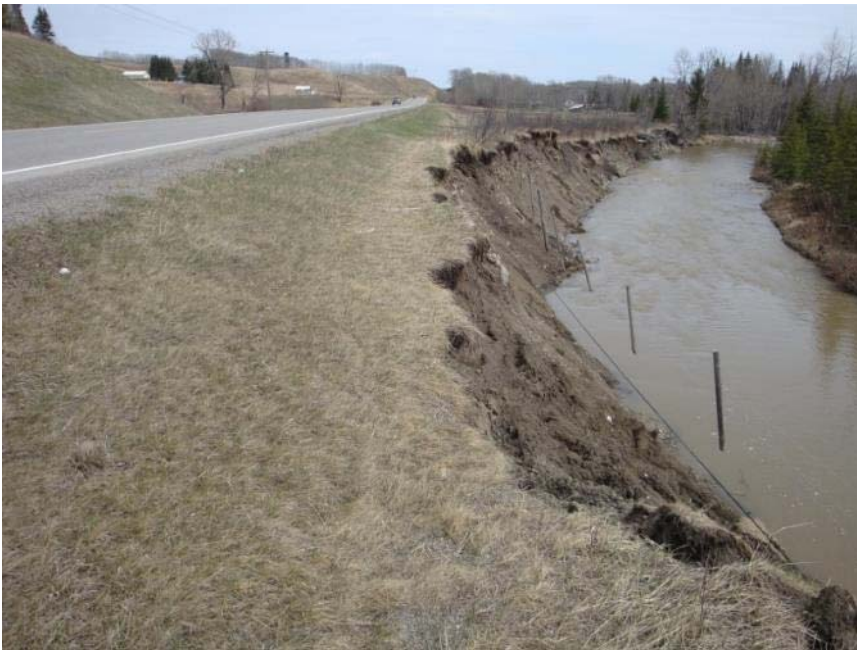
Photo S45-4 (May 2014) – Standing on the bank at the west end of the West Site (similar location to Photo S45-3), looking towards the east at the bank erosion. Note the increased extent of erosion to the east and number of fence posts undermined relative to the 2013 conditions.
