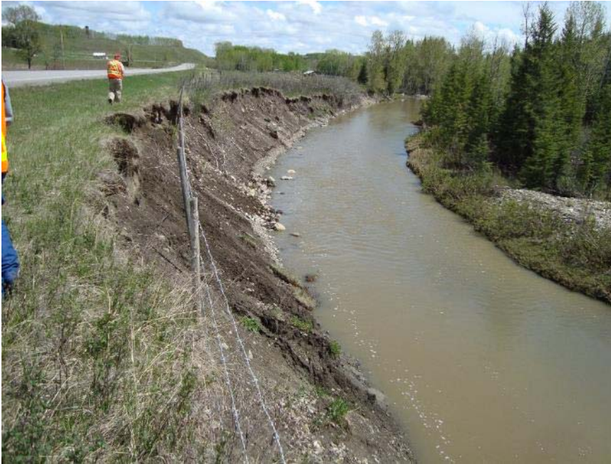
Photo S45-3 (May 2013) – Standing on the bank at the west end of the West Site, looking towards the east at the bank erosion.
