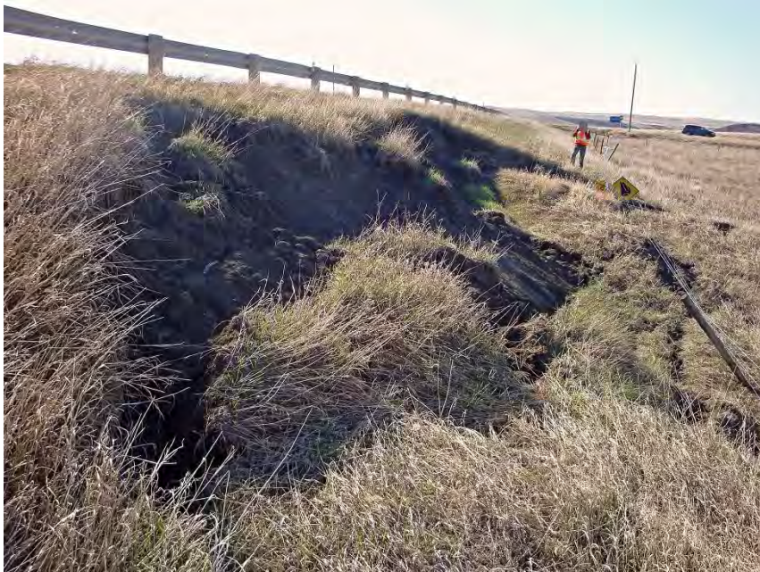
Photo S46-5 (2014) Standing in the same location as the previous photo (S46-4) looking at the Southern Slide. Note the increased downslope movement of the failed soil mass exposing more soil near the headscarp.
