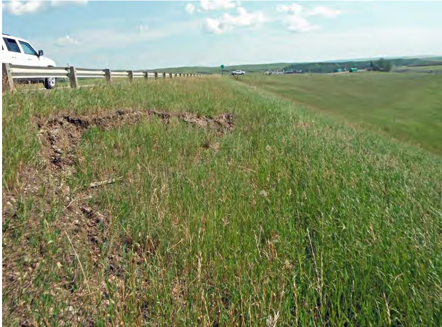
Photo S46-2 (2013) Standing in a similar location to Photo S46-1 and looking to the south at the area referred to as the North Slide during the 2013 inspection. An arc-shaped crack was observed developing within the road embankment. Note that a guardrail has been installed on the west side of the road since 2007.
