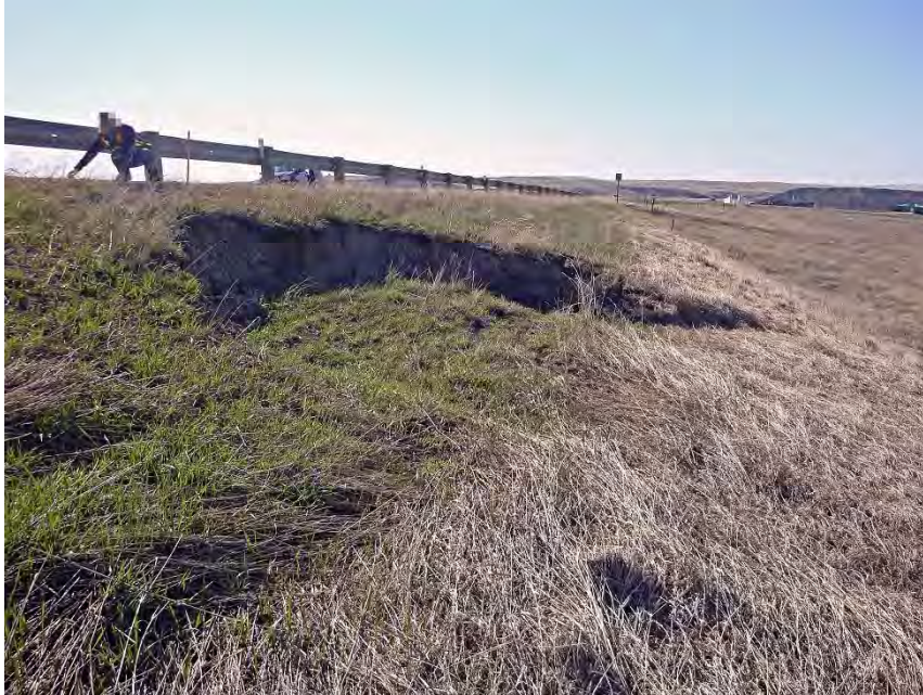
Photo S46-3 (2014) Taken in the same location as the previous photo (S46-2), looking south at the circular earth slide within the road embankment. Note the increased downdrop and downslope displacement relative to the 2013 conditions.
