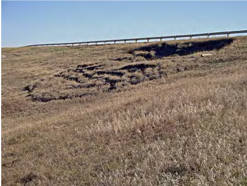
Photo S46-6 (2014) Near the base of the west side of the road embankment looking upslope towards the northeast at the Southern Slide area.
