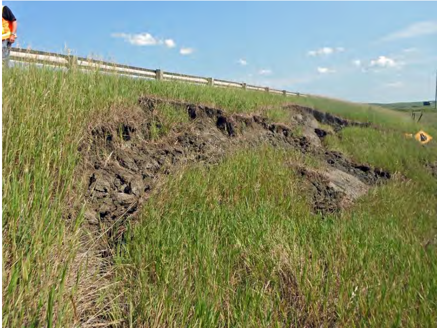
Photo S46-4 (2013) At the Southern Slide area, standing on the west side of the highway embankment looking towards the south at the headscarp of the landslide that formed within the year. Movement is towards the right side of the photo.
