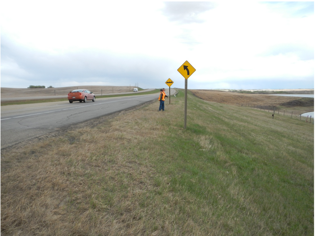
Photograph 1 Pavement Condition May 2013
