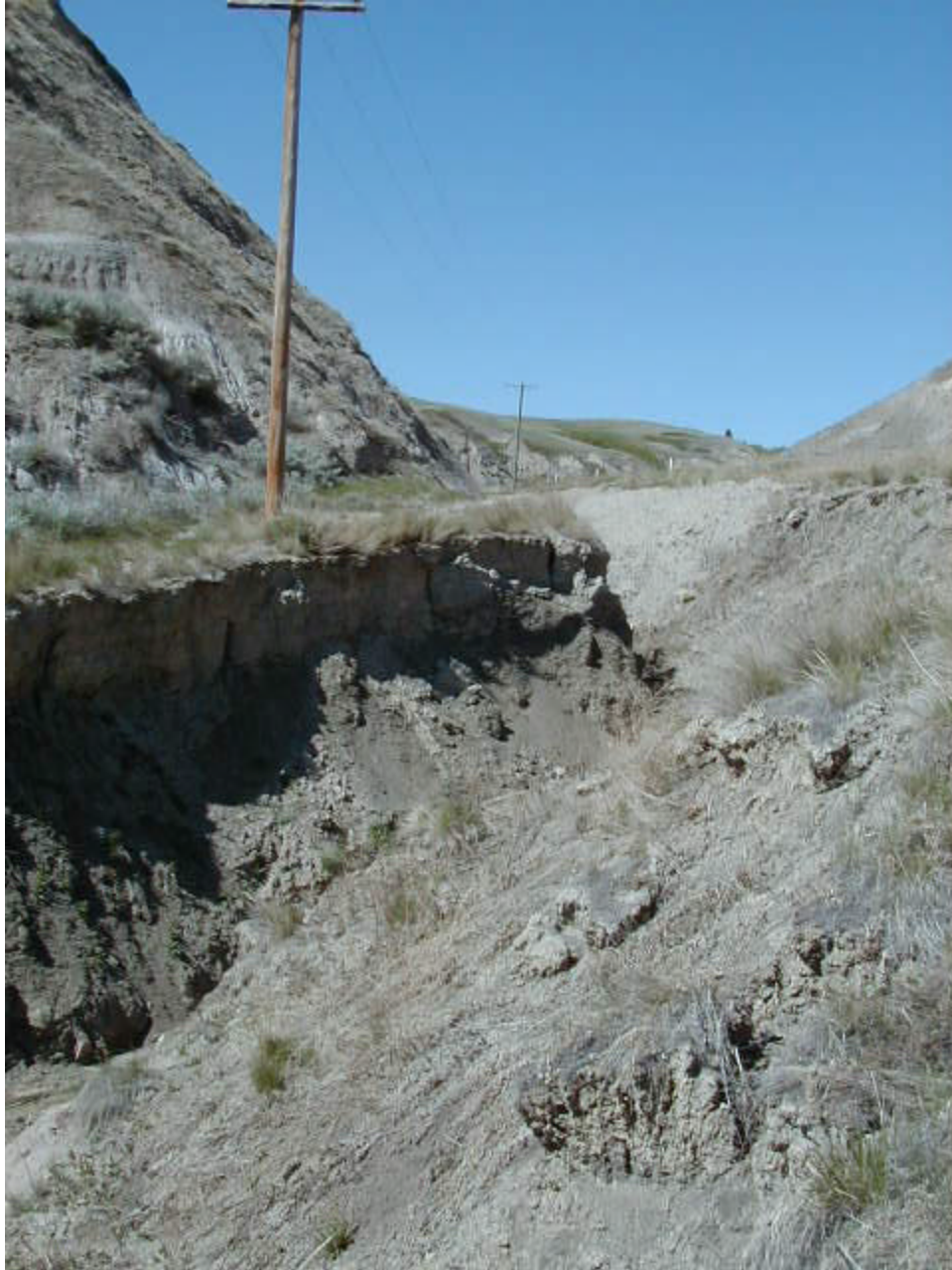
Looking north. Gully is about 5 m deep at power pole.
