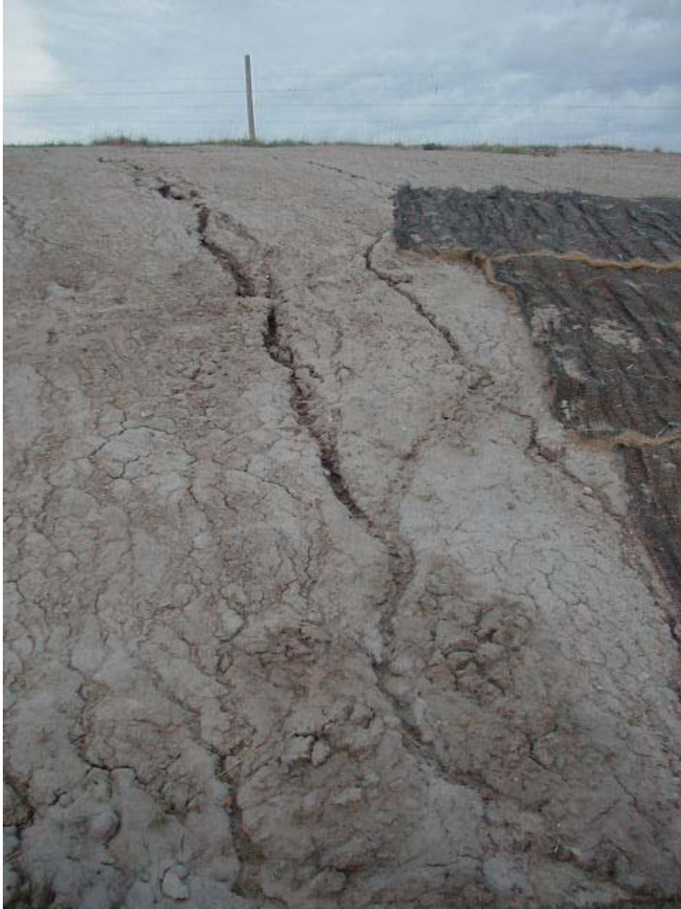
Minor rill erosion beyond matting
