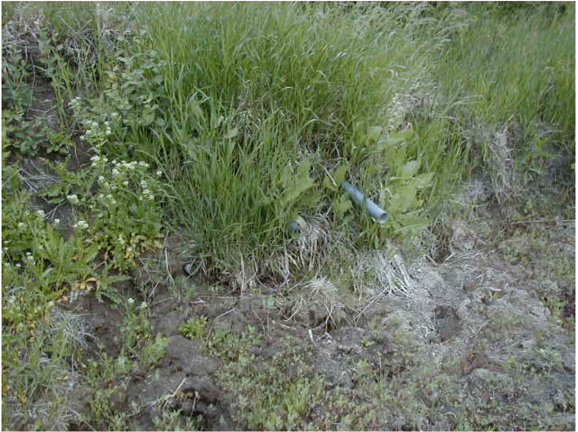
No flow from drains
