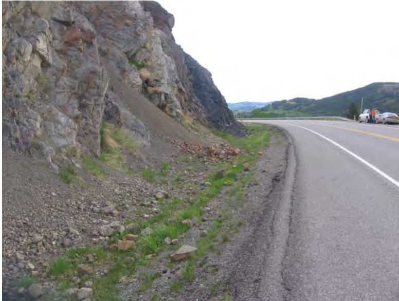
Photo 3 (top) – June 2009 Facing eastbound along the north ditch, showing the accumulation of rockfall debris along the ditch.
