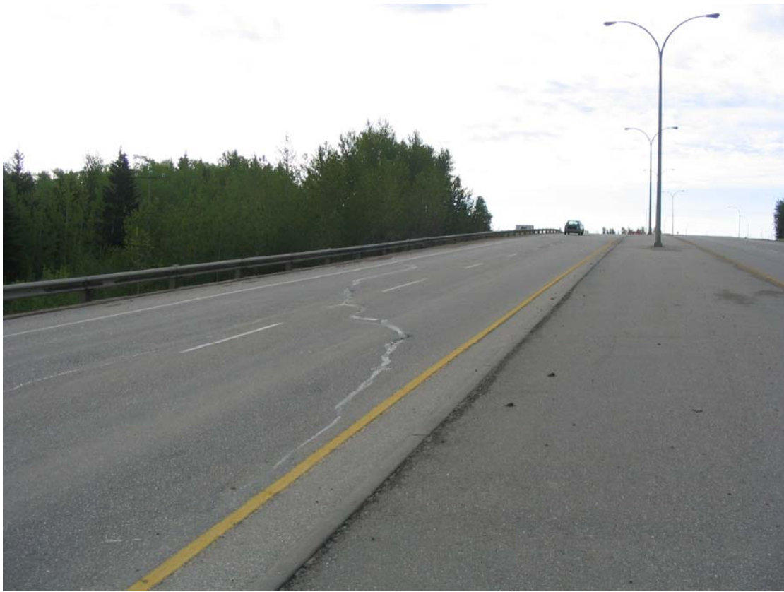
PHOTO 1 EAST CRACK LOOKING WEST
