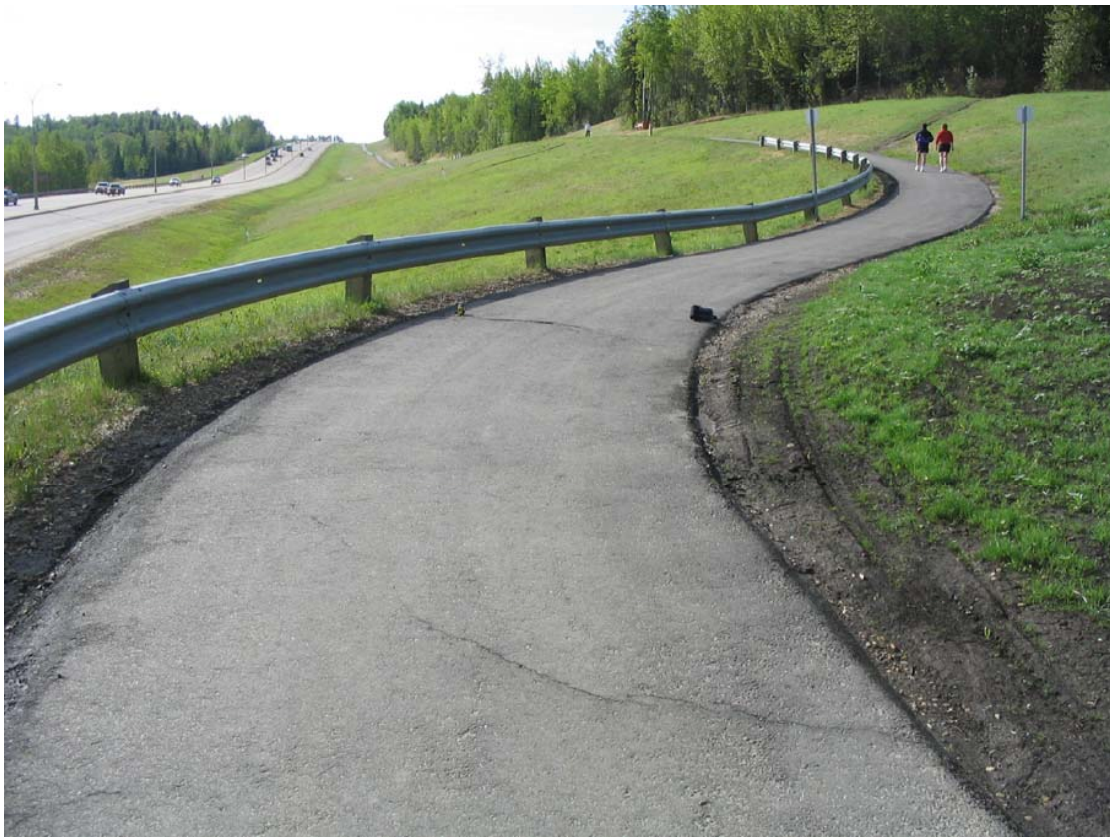
PHOTO 9 TWO EASTERN CRACKS IN NEW ASPHALT TRAIL (LOOKING EAST)
