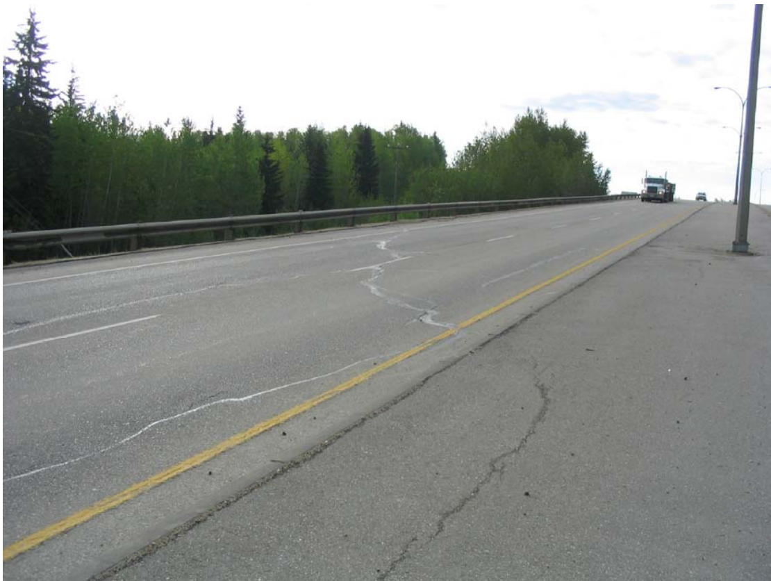
PHOTO 4 WEST CRACK LOOKING EAST
