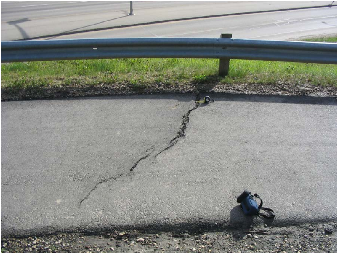
PHOTO 10 EASTERNMOST CRACK IN NEW ASPHALT TRAIL (LOOKING NORTHEAST)
