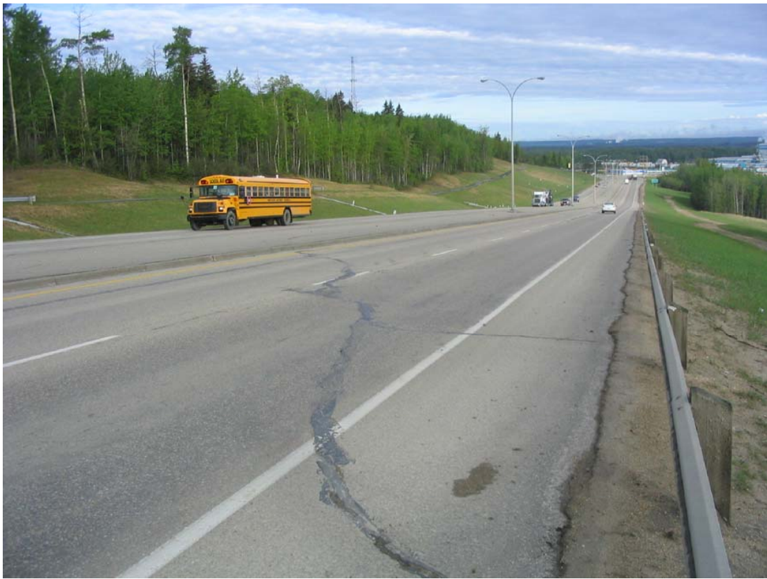
PHOTO 3 WEST CRACK LOOKING WEST
