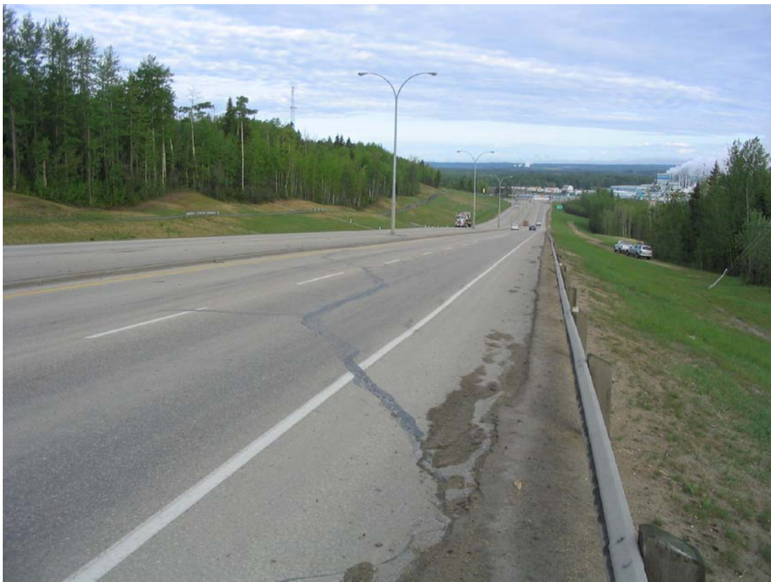
PHOTO 2 EAST CRACK LOOKING EAST
