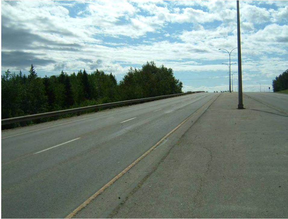
Photo 1 – Looking northeast at west crack, June 5, 2006
