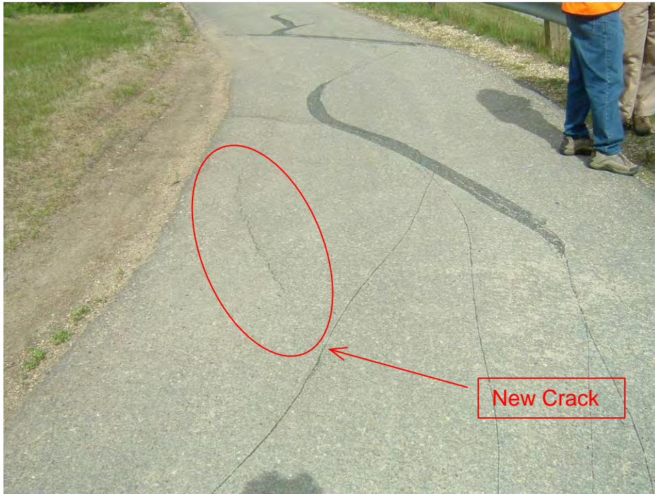
Photo 7 – Closer view of new crack to south of existing cracks, June 5, 2006
