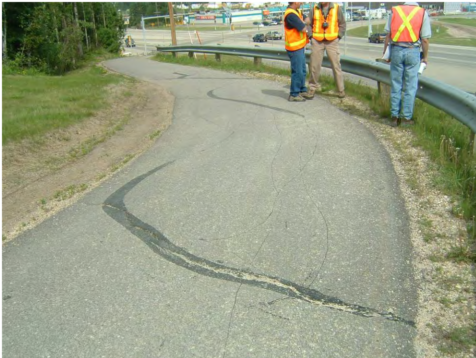
Photo 6 – Looking west at tension cracks in trail above binwall, June 5, 2006
