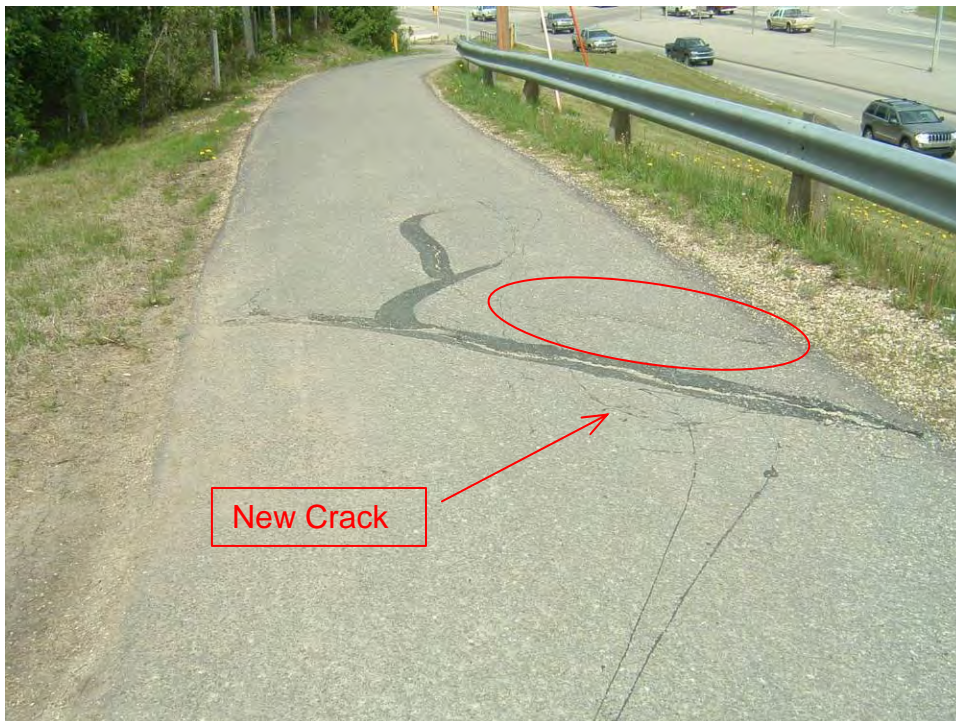
Photo 8 – Closer view of new crack to west of existing cracks, June 5, 2006
