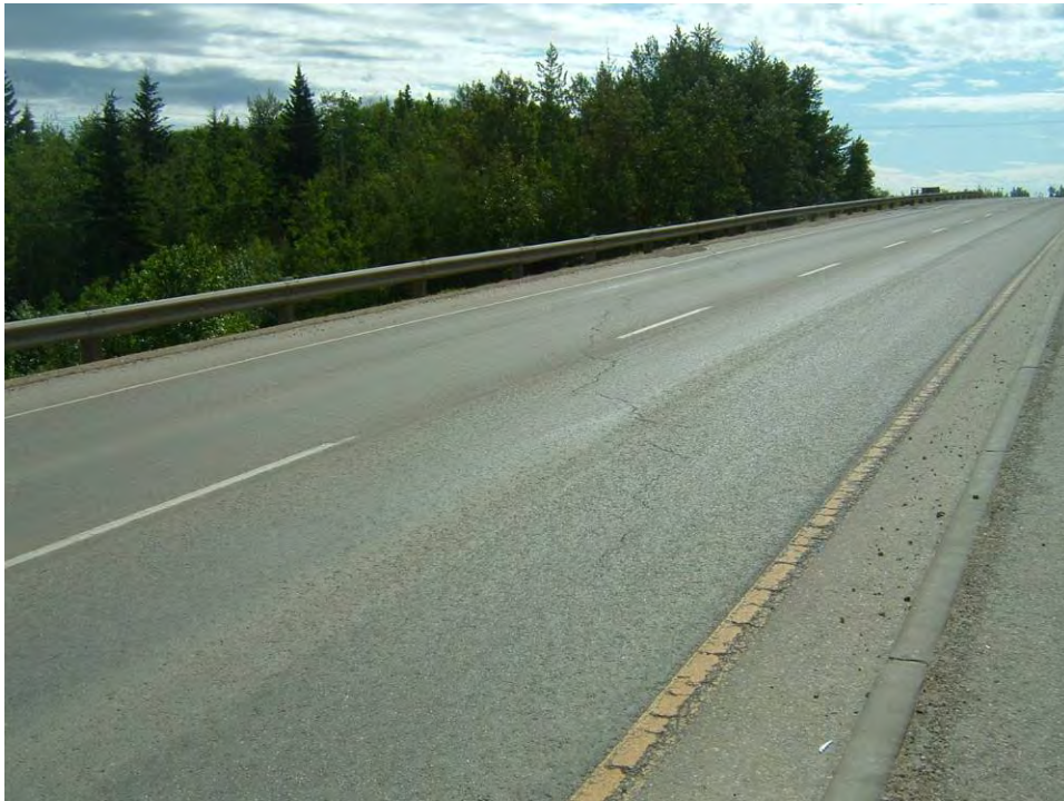
Photo 2 – Looking northeast at east crack, June 5, 2006
