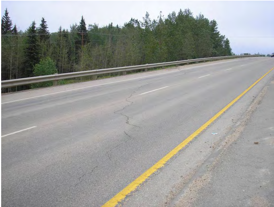
Photo 2 – Looking northeast at east crack, June 11, 2007.
