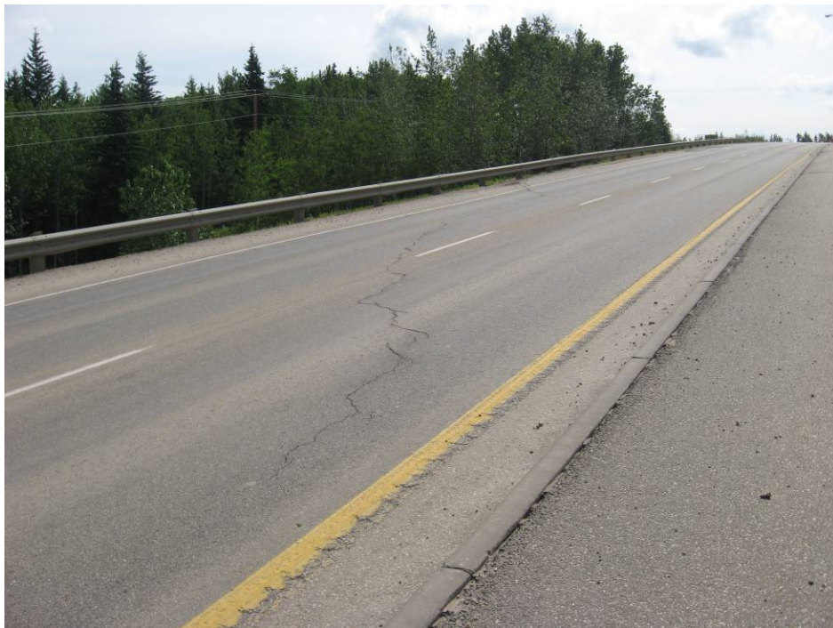
Photo 2 – Looking northeast at east crack, June 11, 2008.
