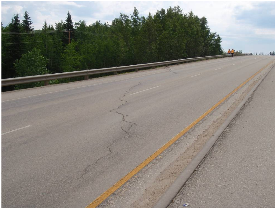
Photo 4 – Looking northeast at east crack (June 15, 2009).
