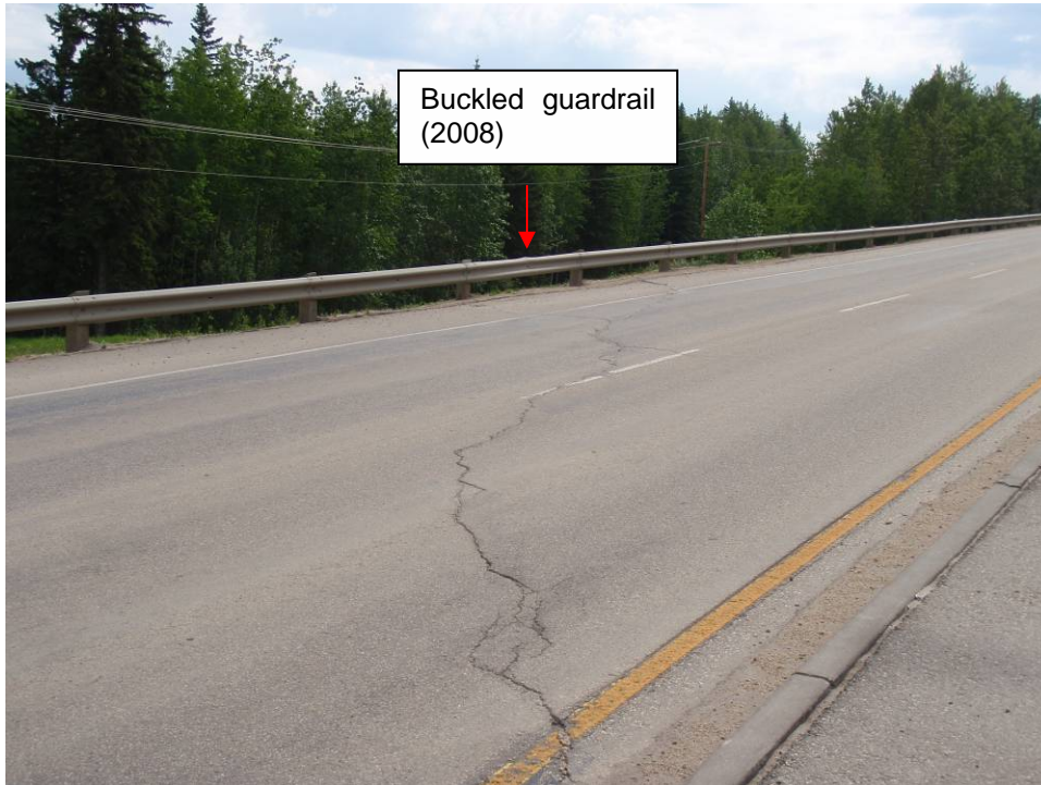
Photo 3 – Looking northeast at west crack (June 15, 2009).
