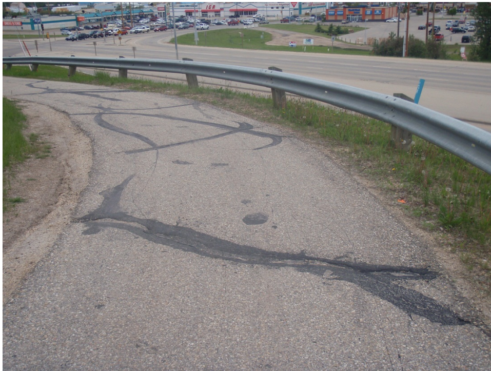
Photo 8 – Looking west at cracks above bin wall. Note tilt of SI30 casing just beyond guardrail (June 15, 2010).
