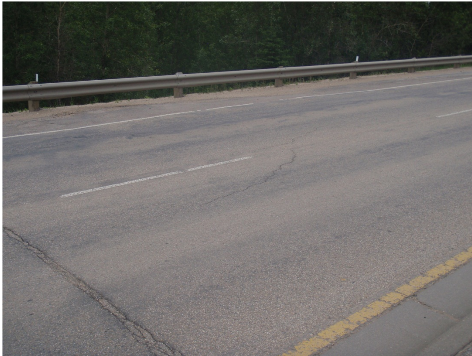
Photo 1 – Looking northeast at catch basin cracks (June 15, 2010).
