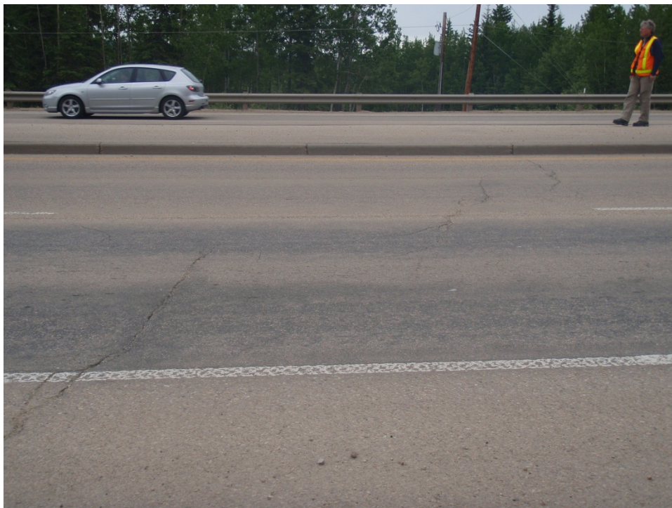
Photo 6 – Looking northeast at culvert dip at Station 1+850 (June 15, 2010).
