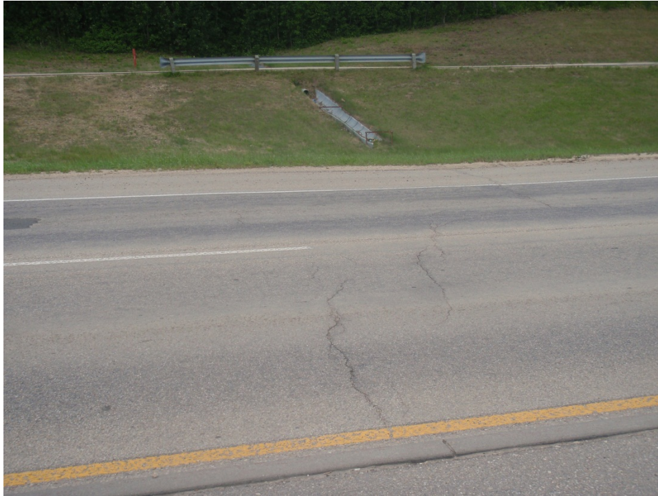
Photo 7 – Gentle dip and pavement crack at Station 1+850 (June 15, 2010).
