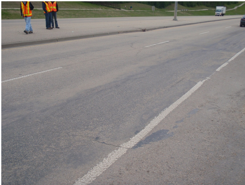
Photo 2 – Looking southwest at catch basin cracks (June 15, 2010).
