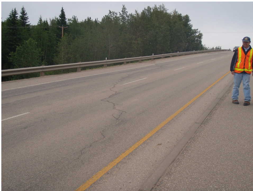
Photo 4 – Looking northeast at east crack (June 15, 2010).
