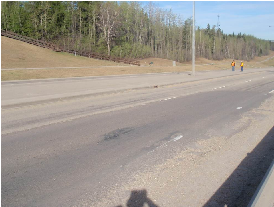
Photo 2 – Looking southwest at catch basin cracks (May 17, 2011).
