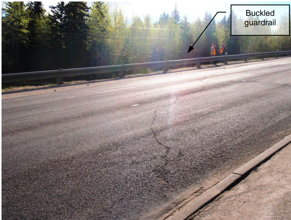
Photo 3 – Looking northeast at west crack (May 17, 2011).
