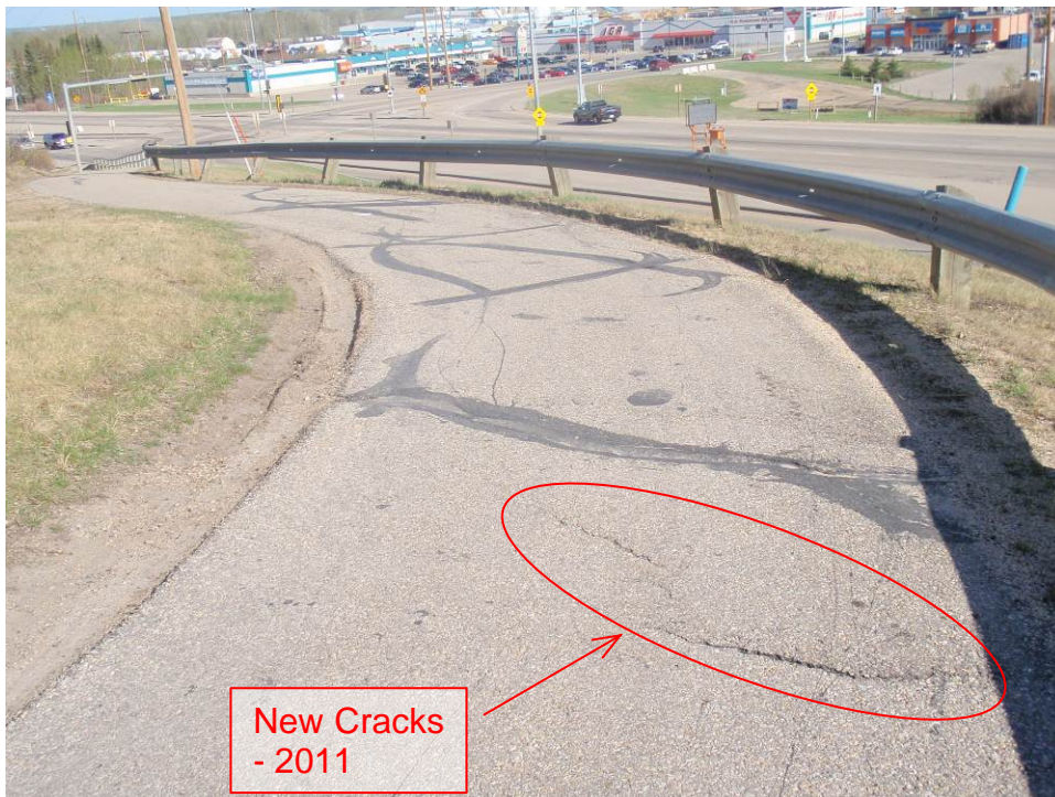
Photo 8 – Looking west at cracks above bin wall. Note tilt of SI30 casing just beyond guardrail (May 17, 2011).
