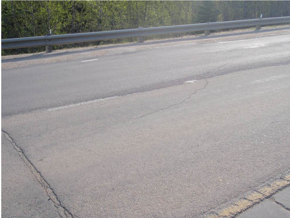
Photo 1 – Looking northeast at catch basin cracks (May 17, 2011).
