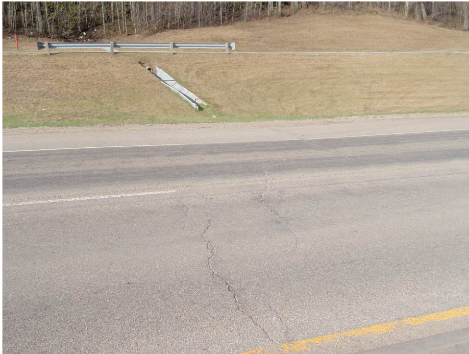
Photo 7 – Gentle dip and pavement crack at Station 1+850 (May 17, 2011).
