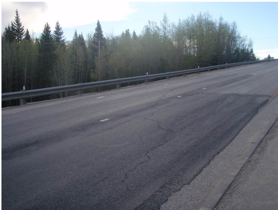
Photo 4 – Looking northeast at east crack (May 17, 2011).
