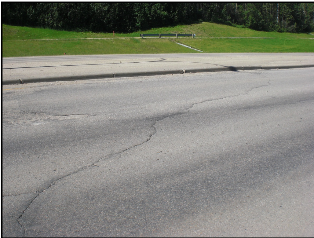
PHOTO 4: West Cracks, facing North.
