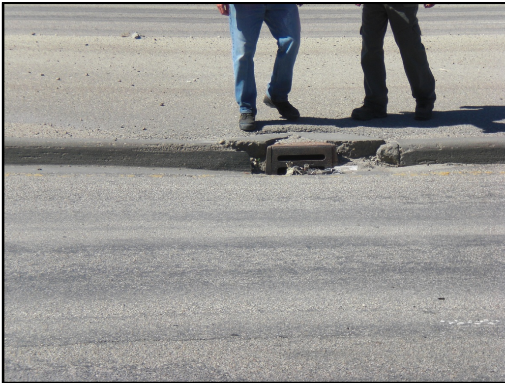
PHOTO 1: Dip in pavement at Catch Basin Cracks.
