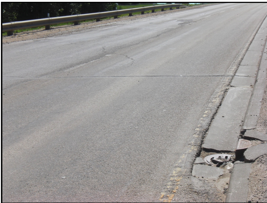
PHOTO 2: Catch Basin Cracks, facing East.
