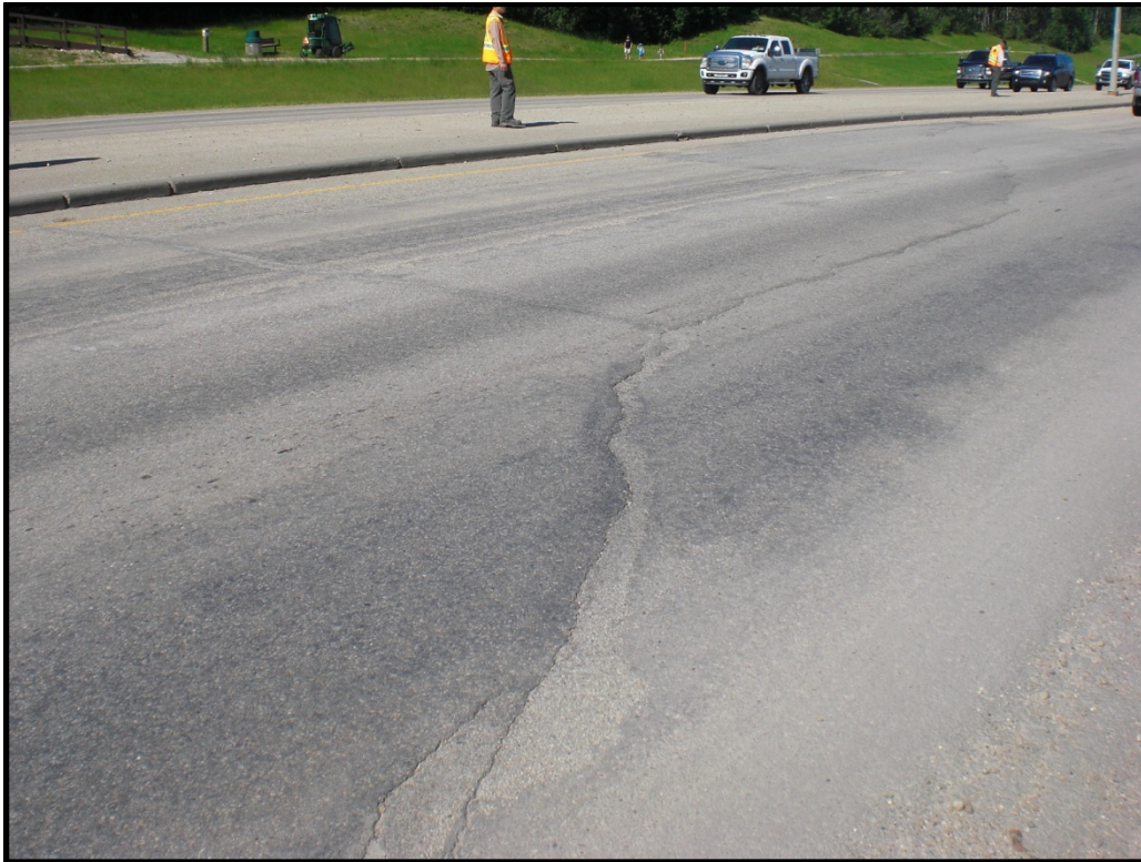
PHOTO 3: East Cracks, facing West.
